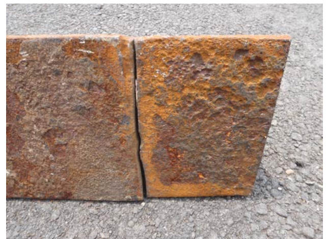
Figure 3: Rust on Underside of the Rail Base
