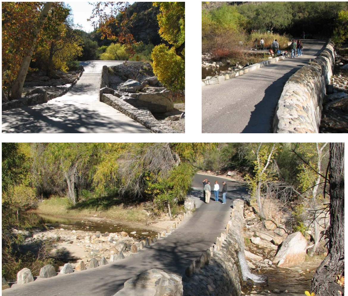
Figure 25 – Bridges of Upper Sabino Canyon Road. Note the decorative 'dragon teeth' in set in the rock masonry (bottom). Courtesy: USDOT Volpe Center.
