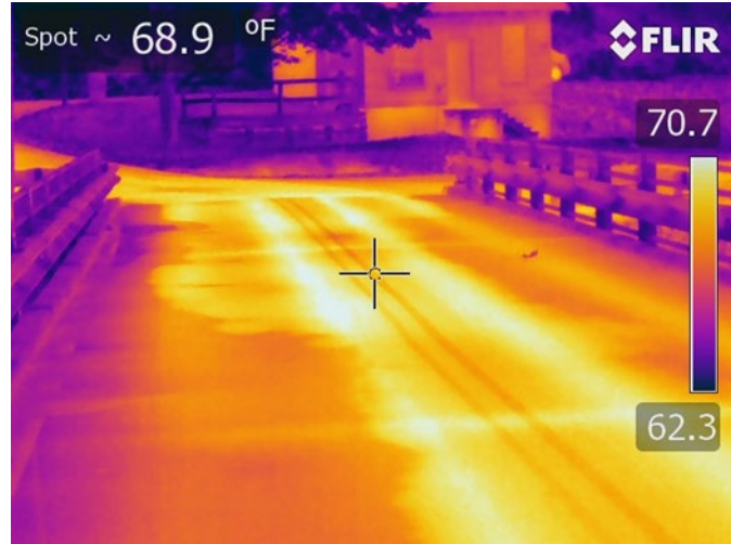
Figure 3.18 FLIR image of Water Pooling Showing Up as Possible Delamination
