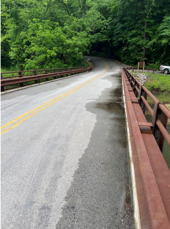
Figure 3.17 Water Pooling in gutter line Following Cold Rain.
