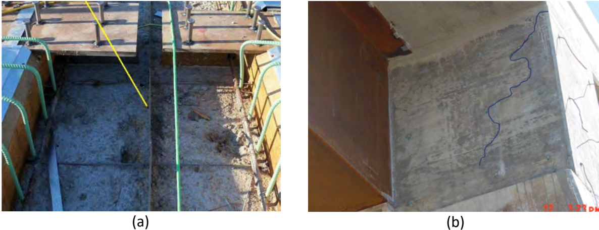
Figure 2-3 (a) Bond breaker plate, (b) uncontrolled cracking in diaphragm [40] .
