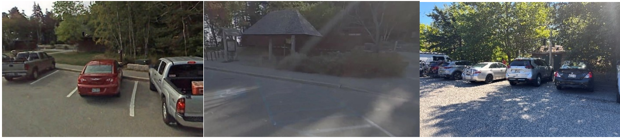
Figure 23: Pavement Marking Degradation 2007, 2019, and 2025
