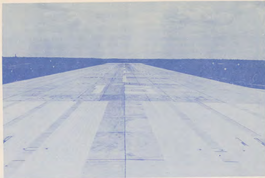
Runway visual aids on runway 13, showing narrow gauge Elfaka and MC-2 lighting configurations.
