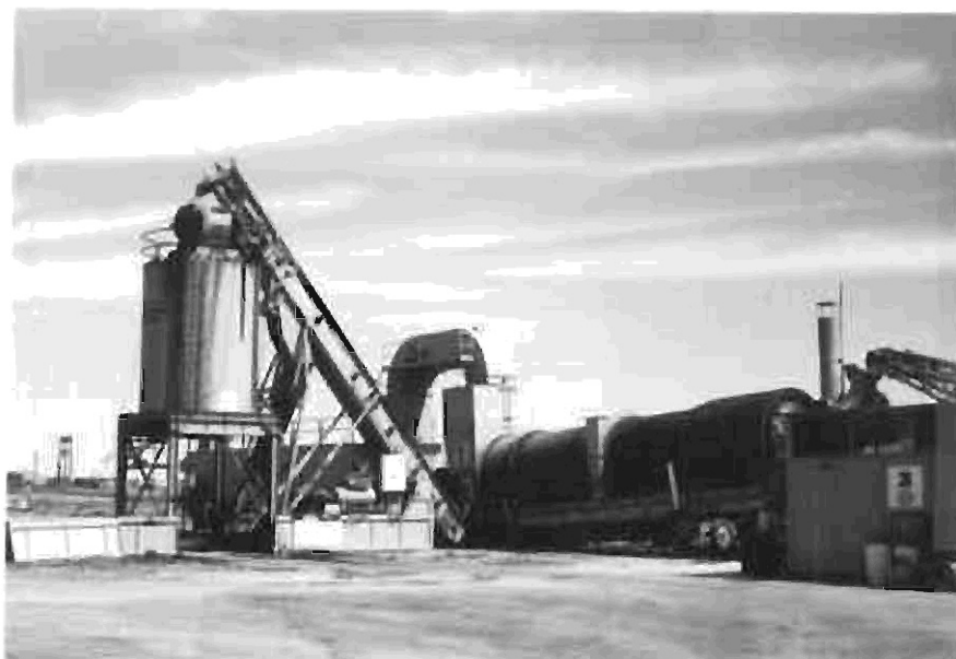
Figure 6. 60-Ton Storage Silo at a Typical Portable Plant
