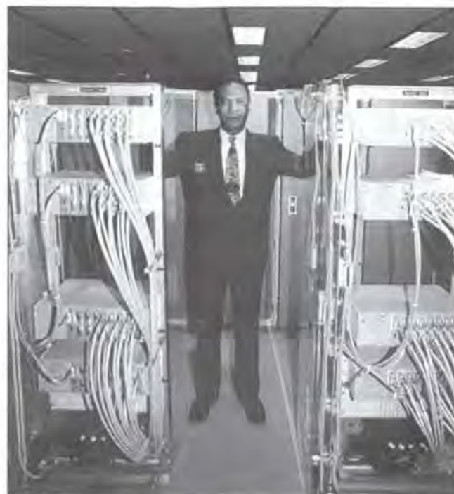
Sam Wilson, site acceptance test lead, with contract traffic simulator unit-CTSU-communications rack.
