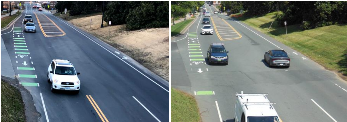
Figure 7. Example of Utility Work Having Removed a Section of Dashed Green-Colored Pavement Markings Without Replacing Them: (left) before utility work; (right) after utility work.
