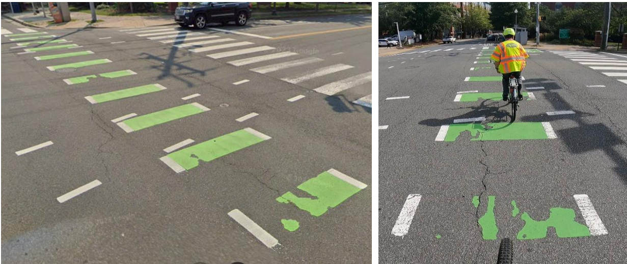
Figure 36. Thermoplastic Green-Colored Pavement Marking Skips at the Clarendon Boulevard and North Rhodes Street Intersection: (left) visible wear in the earliest available Google Maps imaging after installation (image capture: July 2021 © 2026 Google); (right) visible wear to the same skips from a site visit conducted in September 2025
