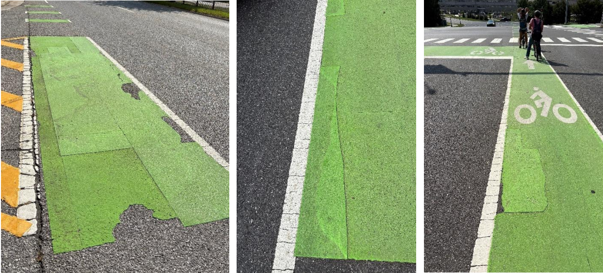
Figure 13. Examples of Marking “Touch-up” Work in Blacksburg with Preformed Green Thermoplastic Placed on Top of Existing Green-Colored Pavement Markings that Had Deteriorated
