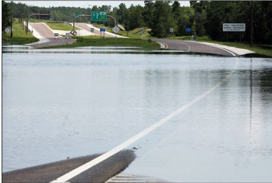
Figure 2. Flooding at Suncoast Parkway in Hernando County, FL (courtesy: Tampa Bay Times /Will Vragovic).
