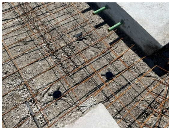
Figure 60. Image. Sensors placed in patch.
