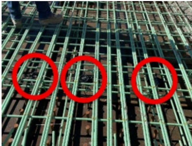
Figure 46. Image. Three sensors placed in bridge deck.
