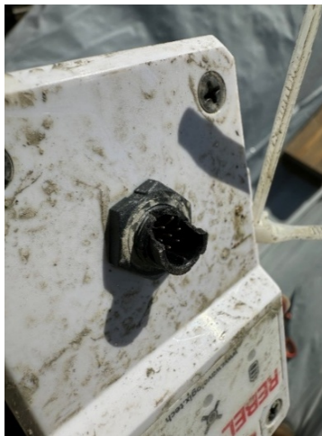
Figure 48. Image. Damaged data logger.
