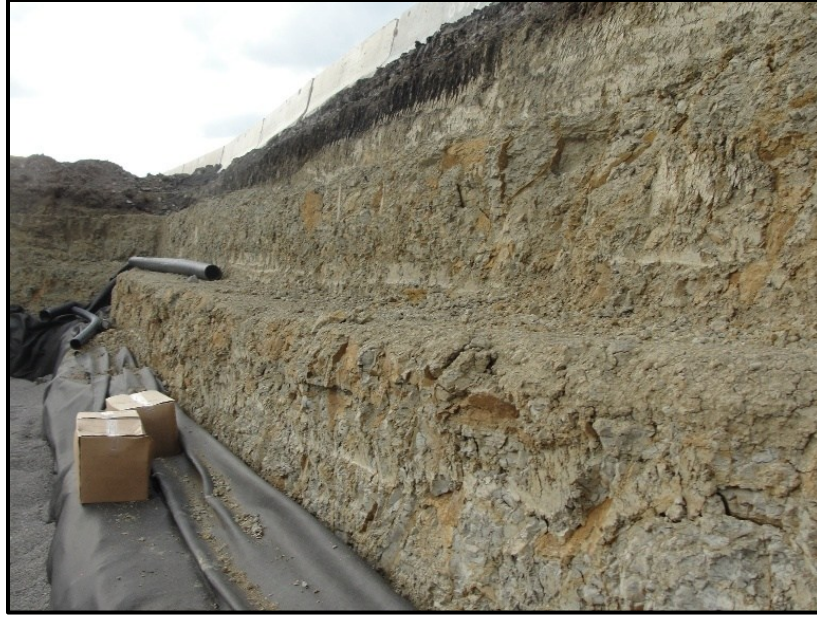
Figure 14. US 50 MP 108 depiction of desiccated clay materials underneath the roadway.
