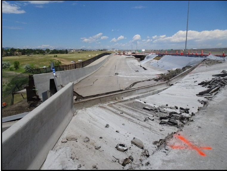
Figure 9 depicts the rigid pavement cracking that occurred in the summer of 2019.
