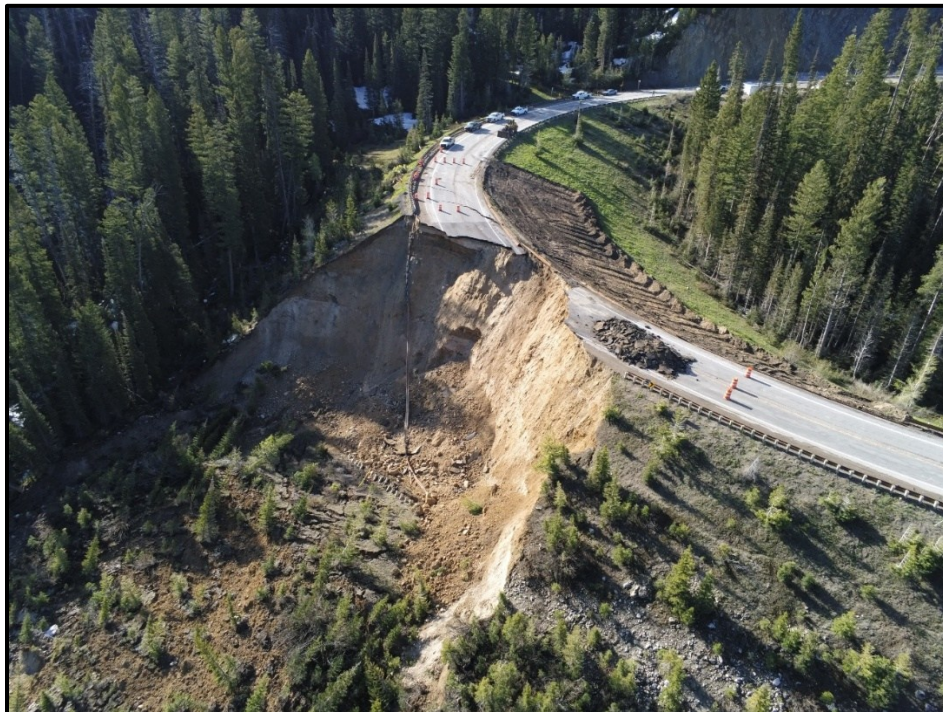
Figure 19. WY 22 MP 12.8 aerial view of embankment landslide failure in 2024.
