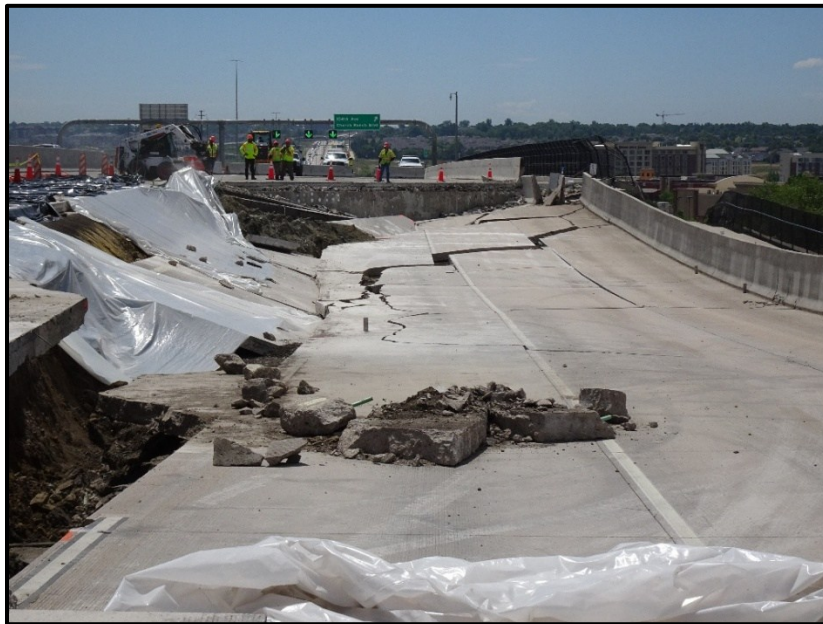
Figure 10. US 36 MP 50.05 depicts the rigid pavement cracking that occurred in the summer of 2019.
