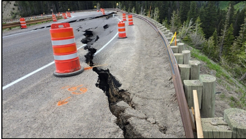
Figure 18. WY 22 MP 12.8 depiction beginning of embankment landslide failure in 2024.
