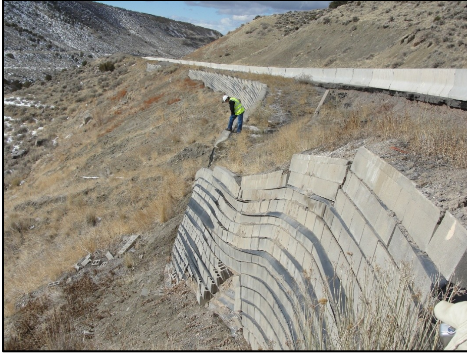
Figure 12. US 50 MP 104.3 depiction of failed block faced wall.
