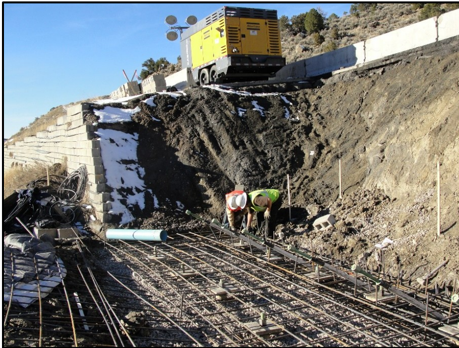
Figure 13. US 50 MP 104.3 depiction of micropiles to support failed block faced wall.
