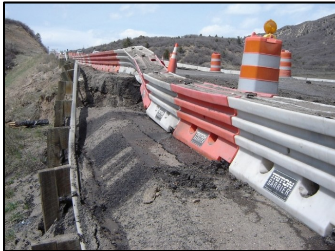
Figure 7. CO 13 MP 15.9 depicts the vertical movement that occurred in just a few days
