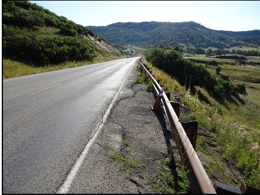
Figure 16. US 84 MP 7.6 depiction of failing roadway shoulder at landslide site.
