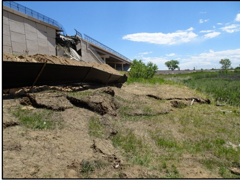
Figure 11 US 36 MP 50.05 depicts the toe of the slope that was failing in bearing/stability, and the toe was overriding the lower surface.
