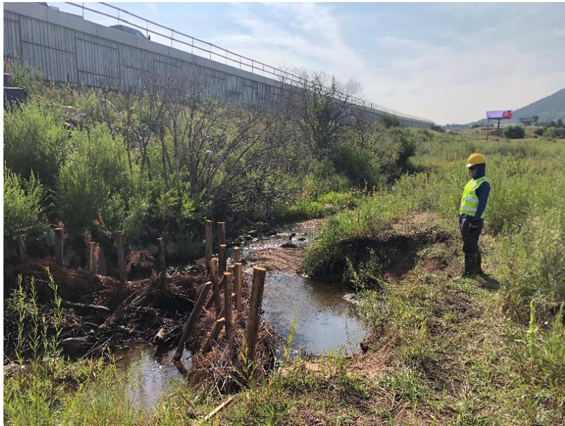
Figure 5. Bank impacts upstream of Interstate 25 along East Plum Creek.
