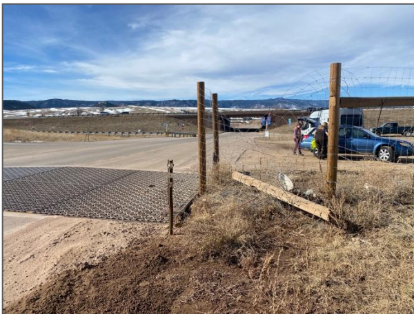
Figure 53. Broken fence post at the Greenland Rd East Wildlife Guard that was down for several months.
