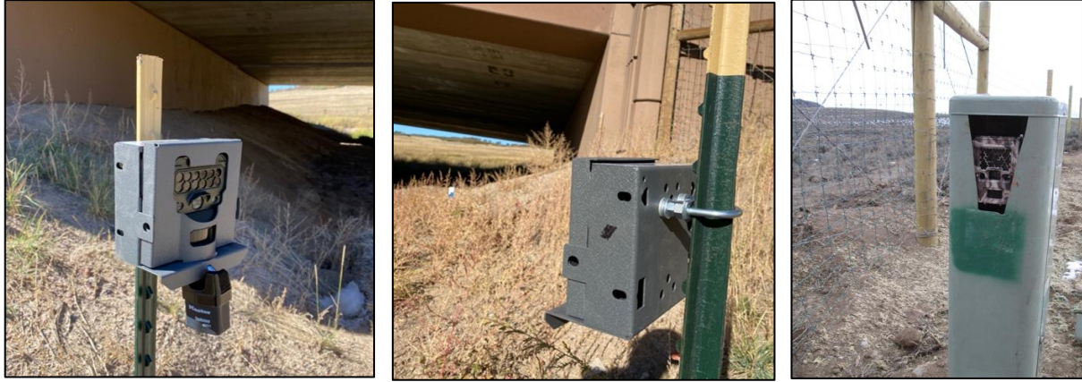
Figure 3. Camera mounted on T-post (left) with U-bolt mounting and security system (middle), and camera mounted in utility box (right).
