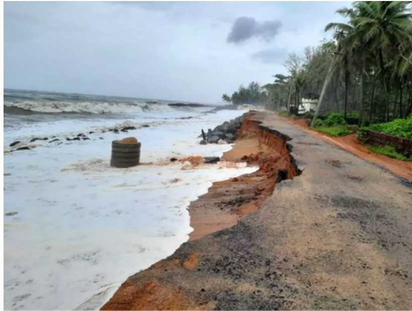
Figure 2. Severe coastal erosion causing partial roadway collapse along the shoreline
