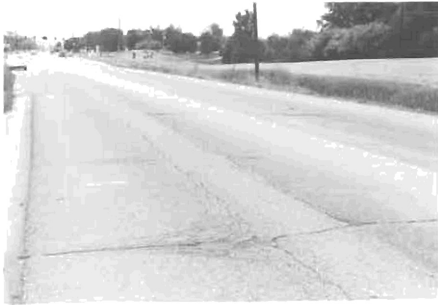
Figure 3. Typical distress found in existing pavement
