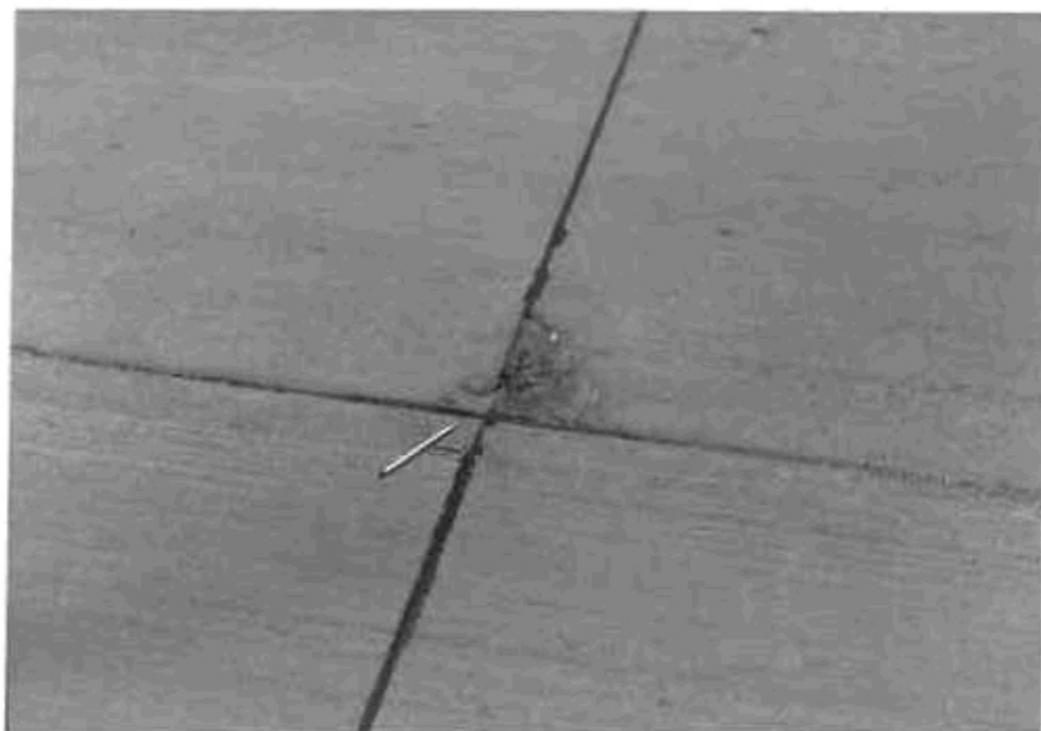
Photo 5&6: Minor corner breaks noted at two locations.
