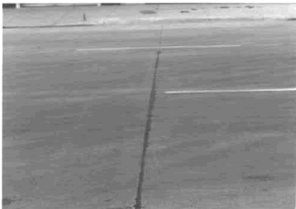
Photo 7: Example of an overfilled joint.
