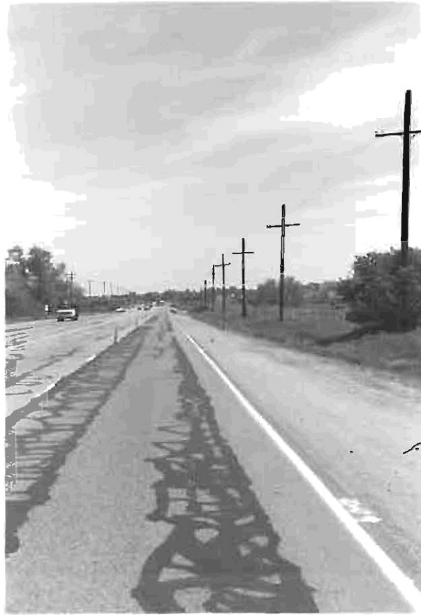
Figure 16. This photograph shows the extent of cracking found on the Santa Fe Drive in Littleton project prior to rehabilitation.
