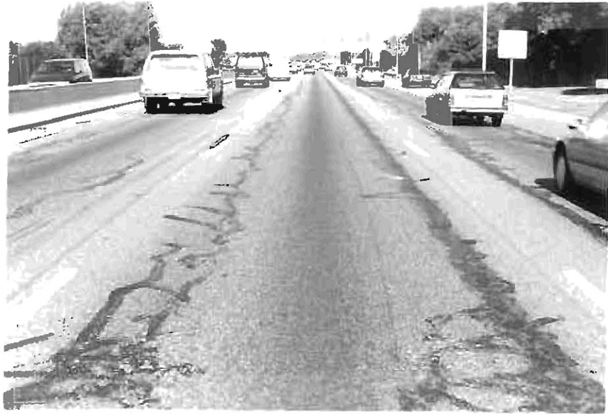
Figure 14. This photograph shows the extent of cracking found on the I-25 in Denver prior to rehabilitation.
