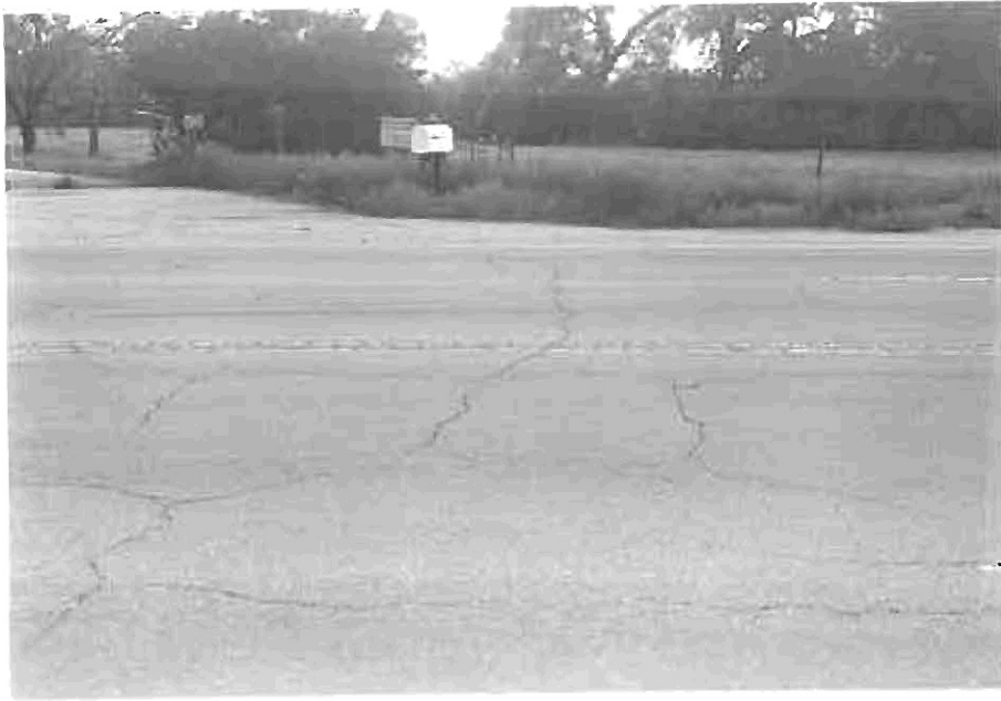
Figure 2. Typical cracking pattern found prior to construction on the Santa Fe Drive project.
