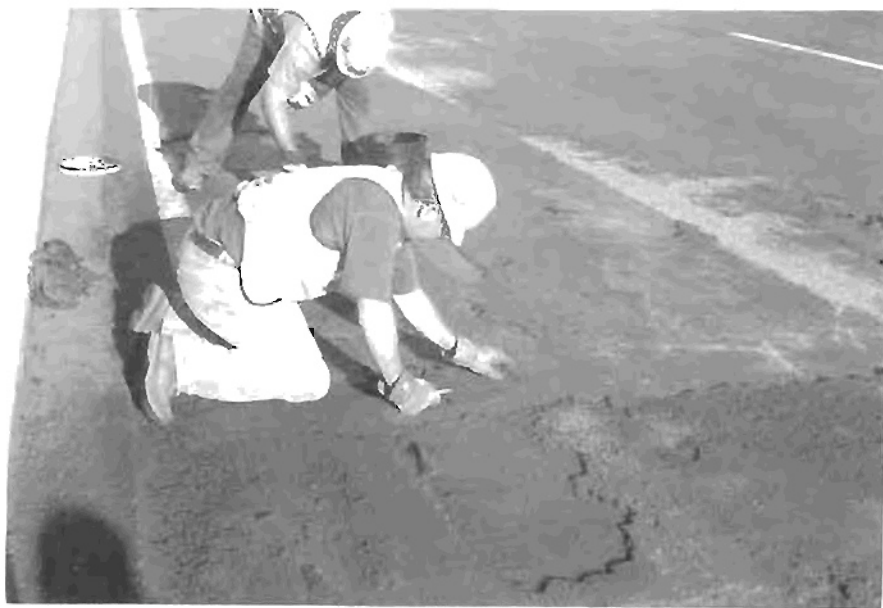
Figure 19. The exposed membrane was removed.
