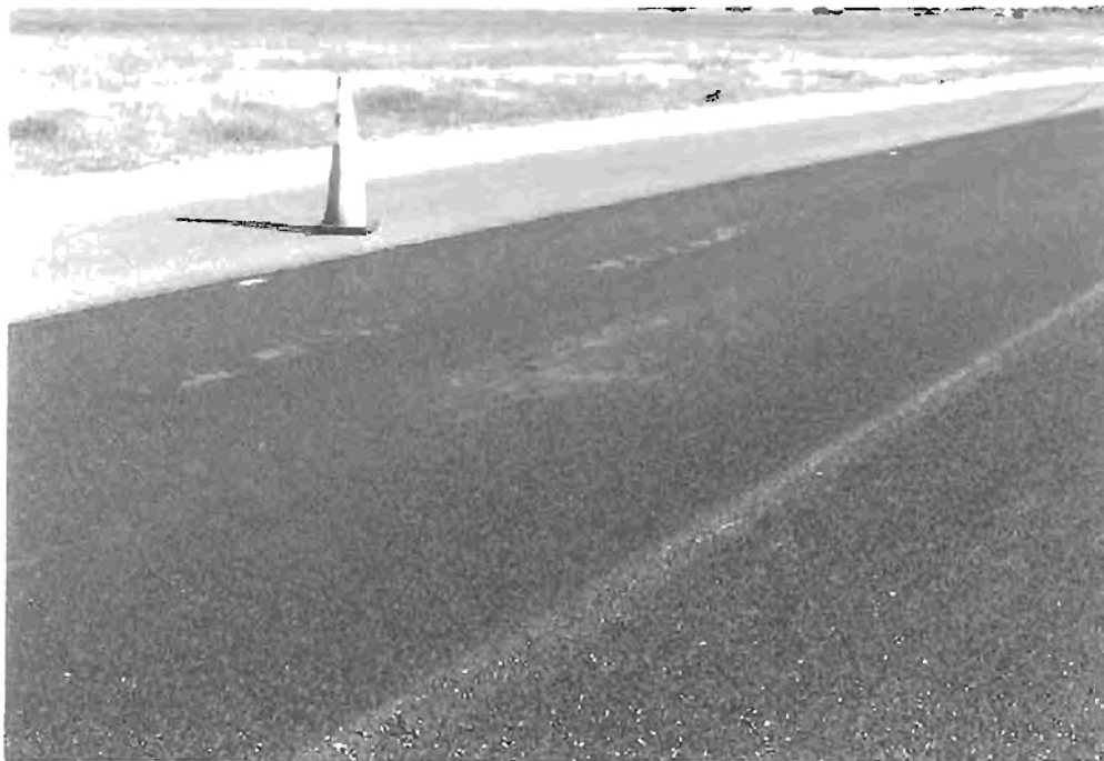
Figure 11. Limited problems with draindown were encountered.
