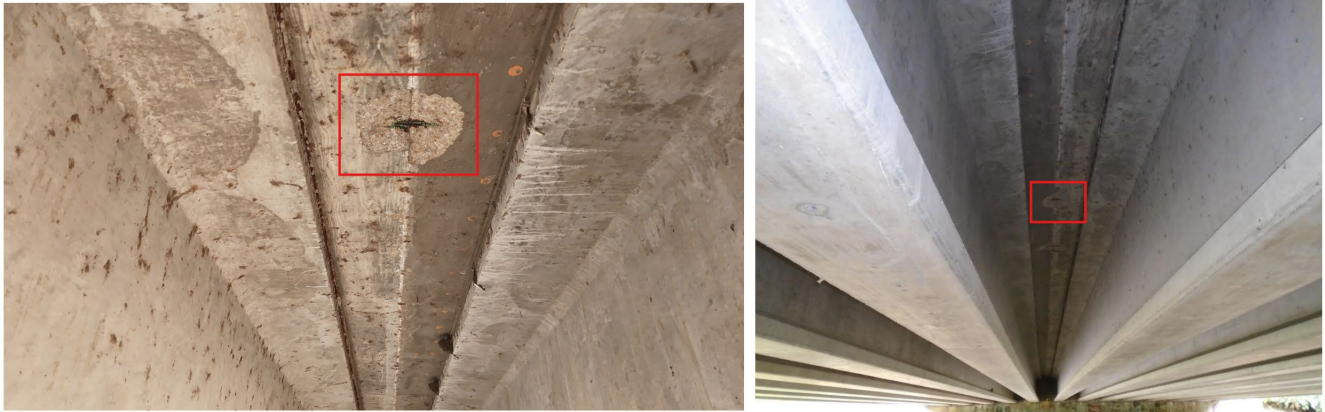
Figure 35. Photo. Comparison of a UAS-collected image (left) and a photograph from a previous inspection (right) showing concrete spalling and exposed rebar on Bridge No. 0580128.
