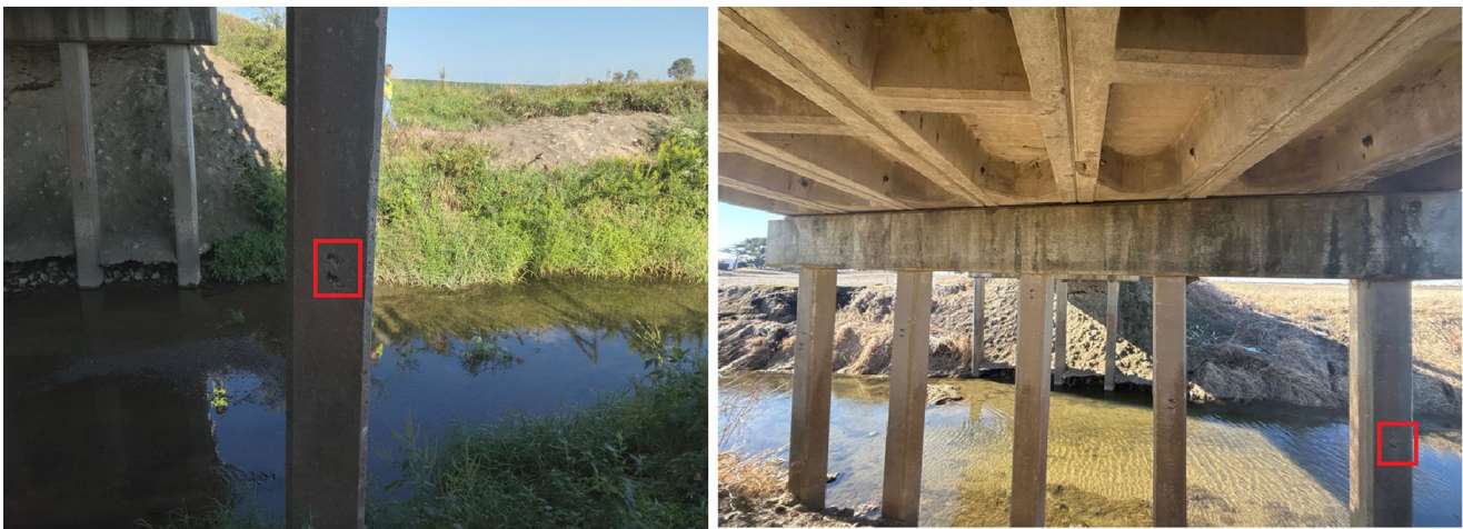
Figure 32. Photo. Comparison of a UAS-collected image (left) and a photograph from a previous inspection (right) showing column spalling on Bridge No. 0103277.
