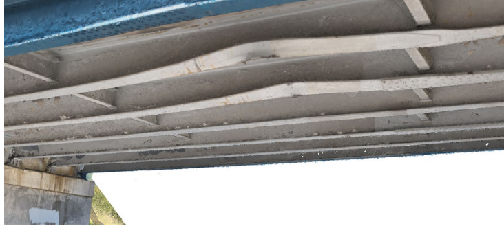
(a) Bottom-side view of the deformed girders
