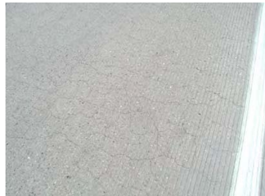
Fig. C.7.7 Cracks on the deck slab
