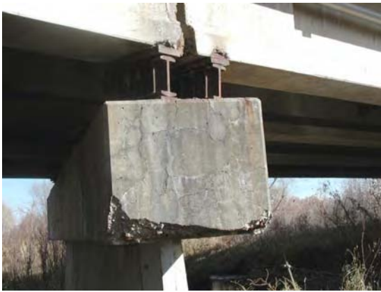
Fig. C.2.5 Spalling on the pier cap
