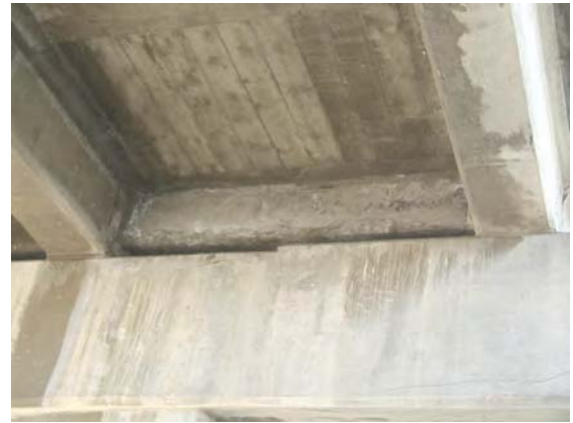
Fig. C.6.9 Severe spalling on the sub-beam
