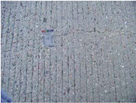
Fig. C.6.8 Transverse crack with width varying from 0.016-0.030 in
