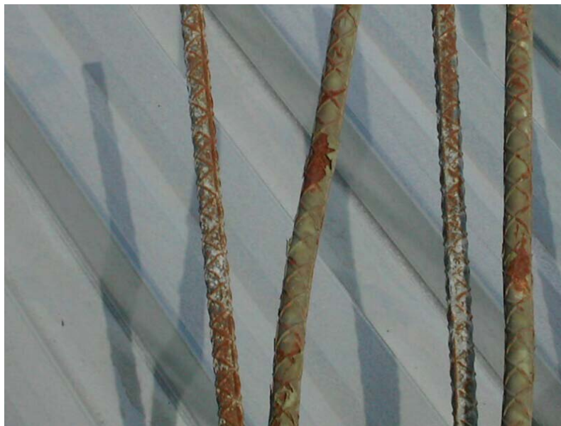
Fig. B1.1.2 Corrosion of epoxy-coated rebars
