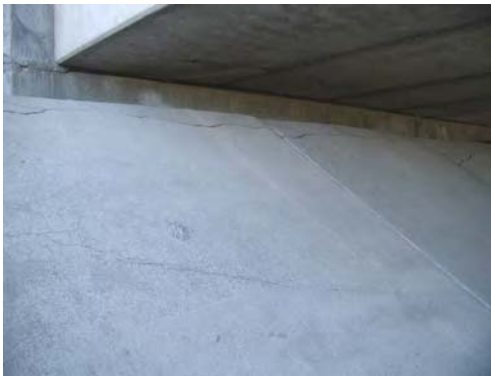
Fig. C.3.10 Cracks around the bridge abutment
