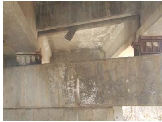
Fig C.2.6 Efflorescence on the bottom and pier cap
