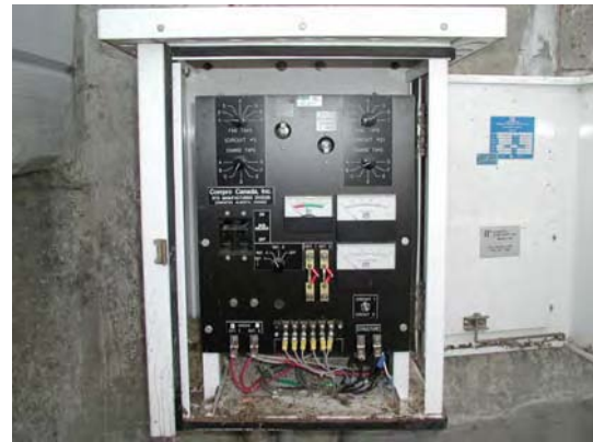
Fig. C.6.5 The control box for the cathodic protection system
