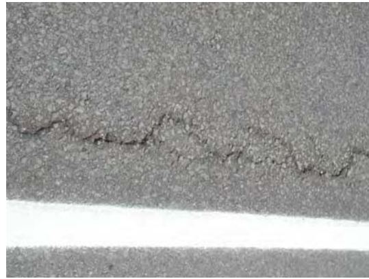
Fig. C.8.5 A longitudinal crack on the asphalt overlay
