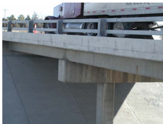
Fig. 1.2 Corrosion damage on pier caps
