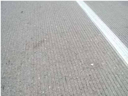
Fig. C.7.6 Cracks on the deck slab
