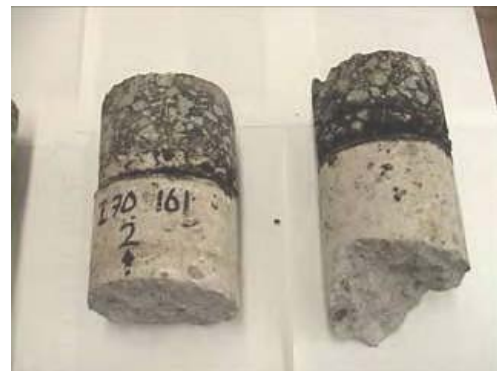
Fig. C.8.12 Concrete cores taken from the driving lane
