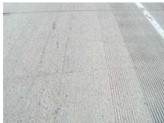
Fig. C.6.7 The transverse cracking
