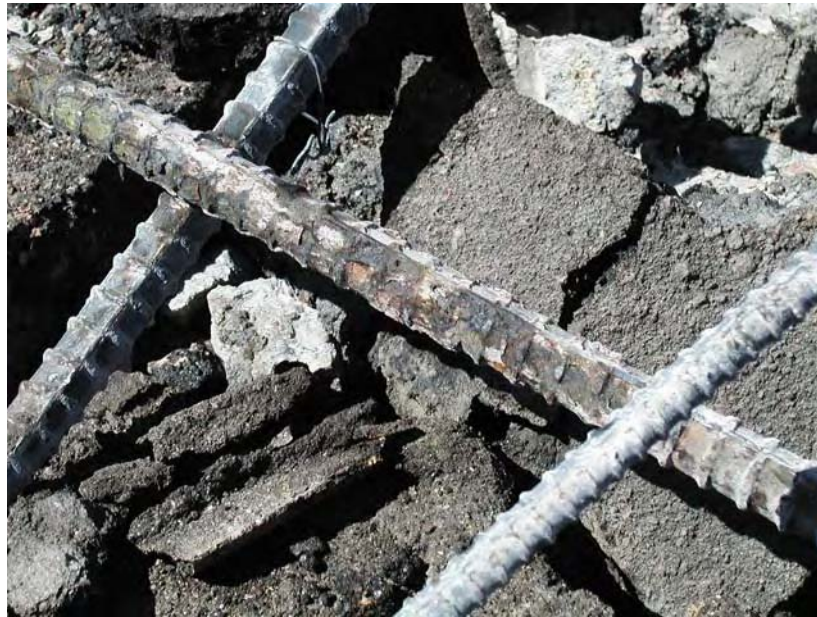
Fig. B1.7.7 Corrosion of steel bars
