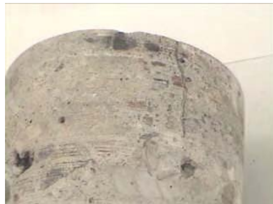
Fig. C.3.13 Cracking in the core
