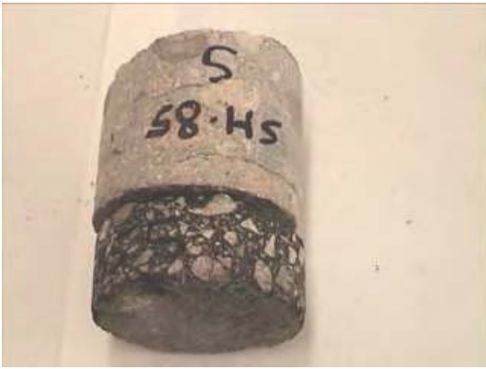
Fig. C.1.12 Cracking in the core – shoulder lane
