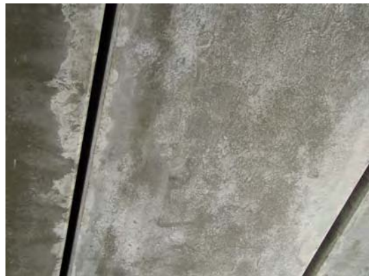
Fig. C.3.7 Efflorescences at the bottom of bridge decks
