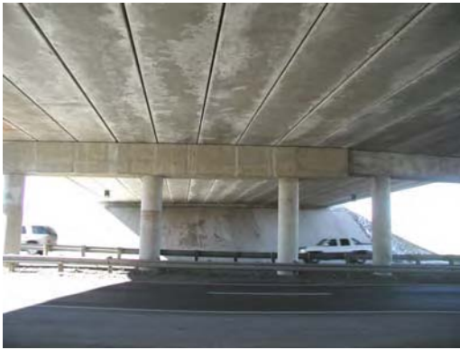
Fig. C.3.8 Efflorescence on the bottom deck
