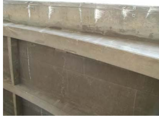
Fig. C.8.9 Efflorescence on the shoulder
