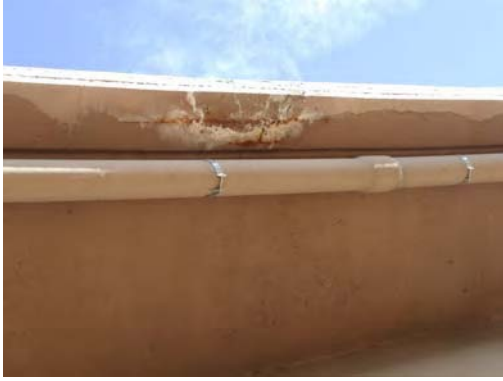
Fig. C.9.4 Efflorescence on the overhang structure
