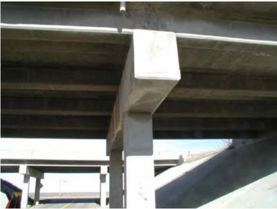
Fig. C.6.10 Cracks on a pier cap
