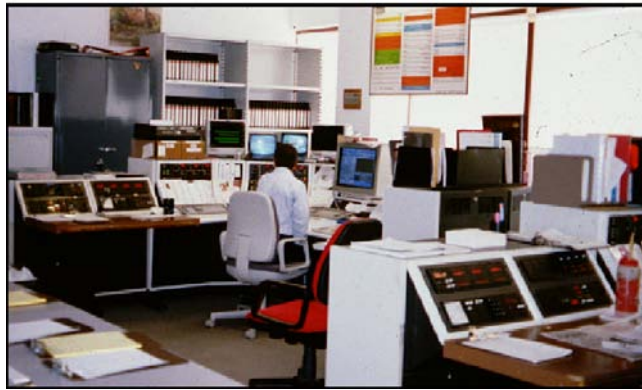
Figure A-9 New Dispatcher's Console
