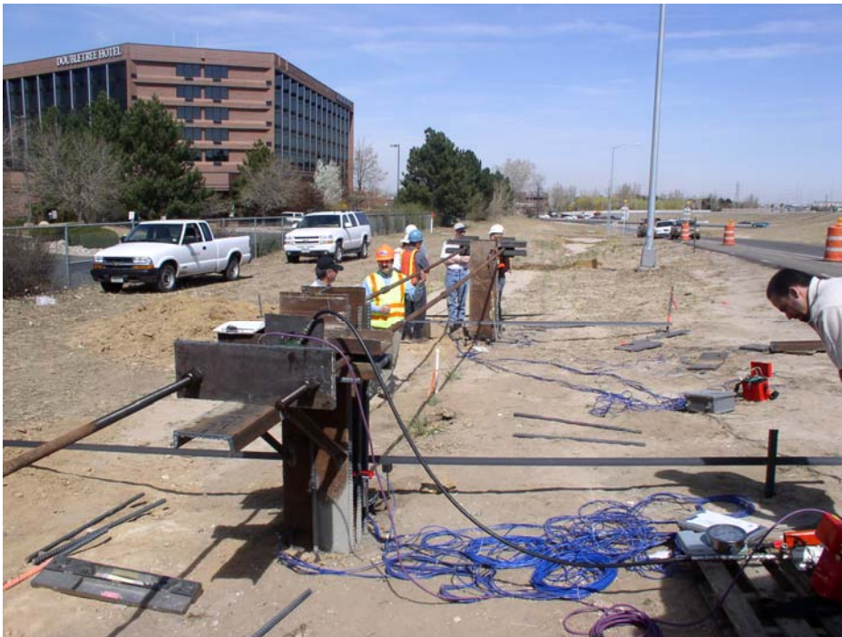
Figure 5.52 Running the test and watching the instruments
