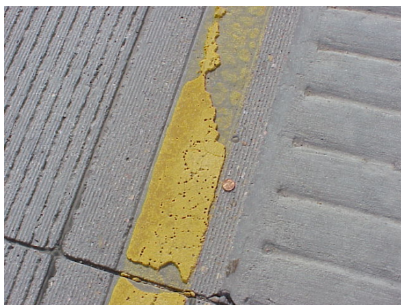
Figure 7. The thermoplastic failed due to adhesion loss.
