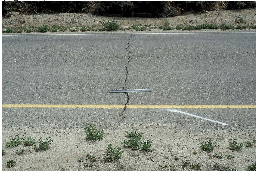
Figure 19 - High Severity Transverse Cracking
