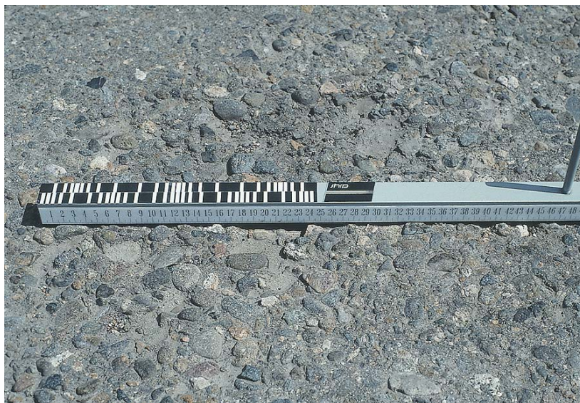
Figure 31 - Loss of Course Aggregate
