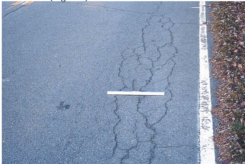
Figure 4 - Moderate Severity Fatigue Cracking
