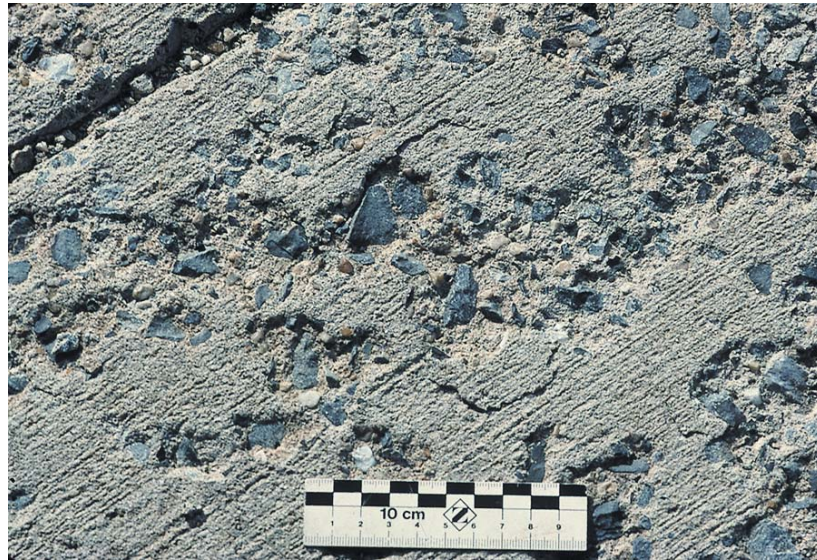
Figure 54 - Scaling, Close-up View
