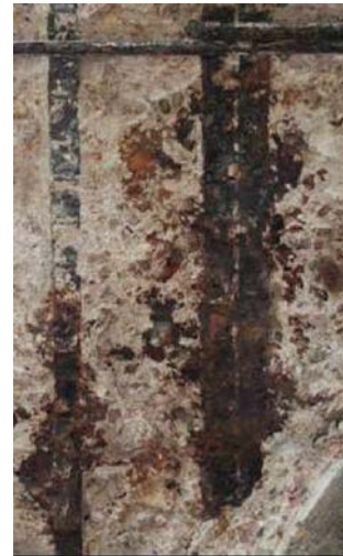
Figure 2-4 The corrosion in arch
