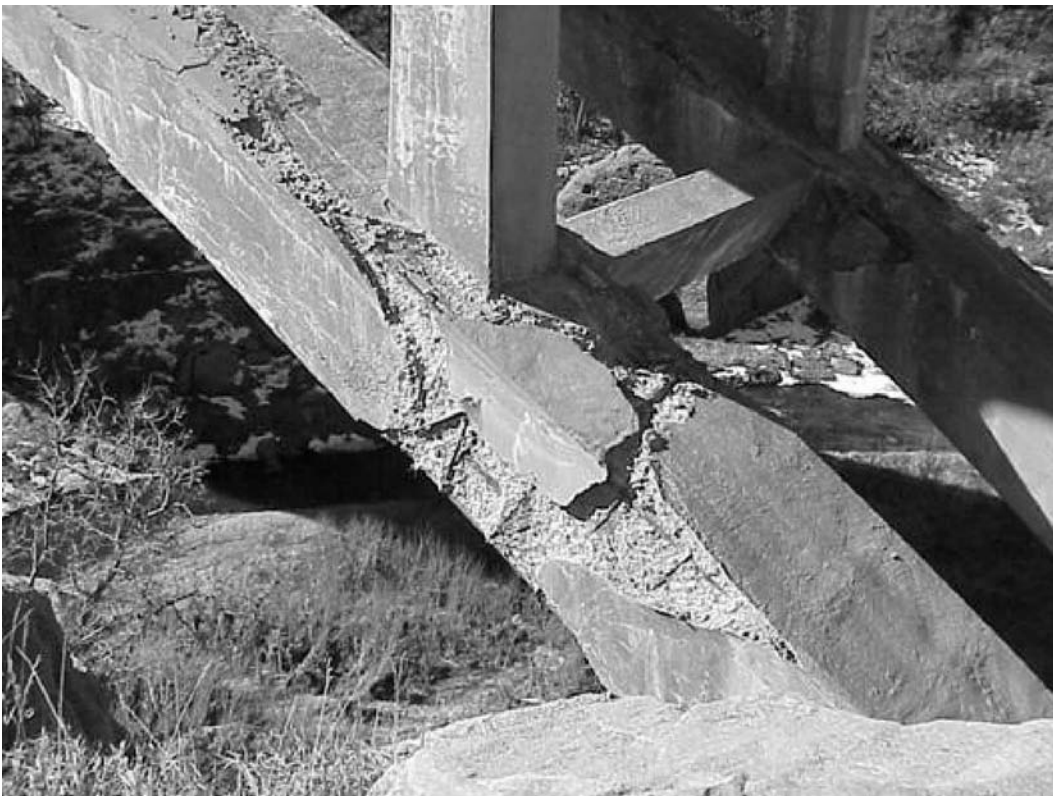
Figure 1-3 Spalling concrete and exposed steel before repair
