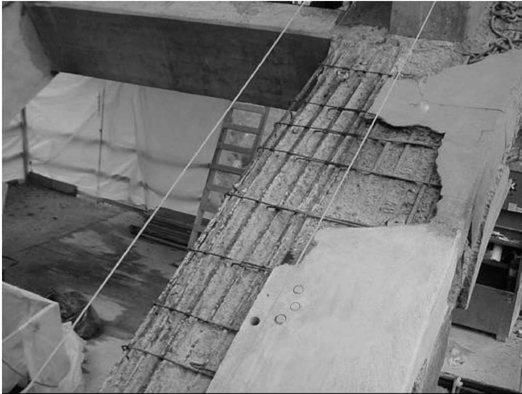
Figure 1-4 Spalling concrete and exposed steel during construction
