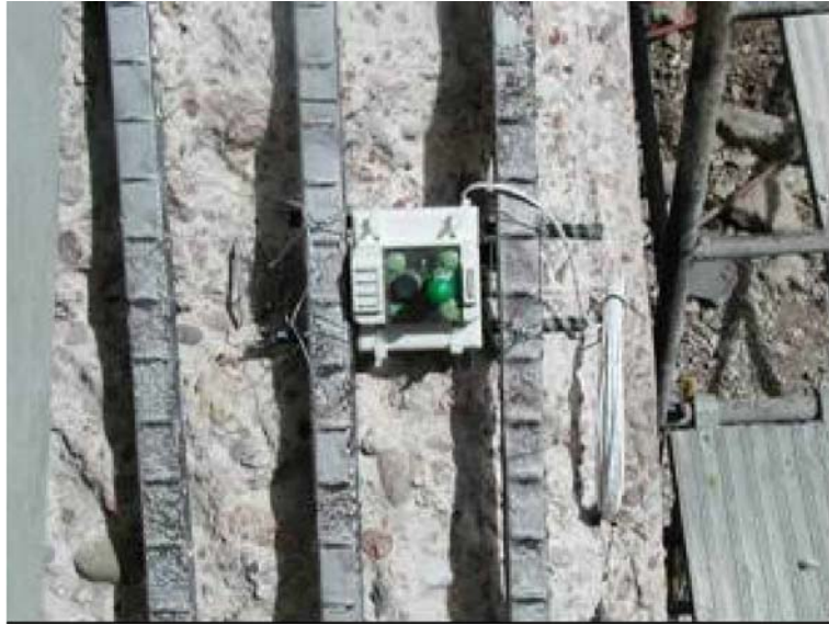
Figure 3-10 An installed corrosion sensor (ECI-1)
