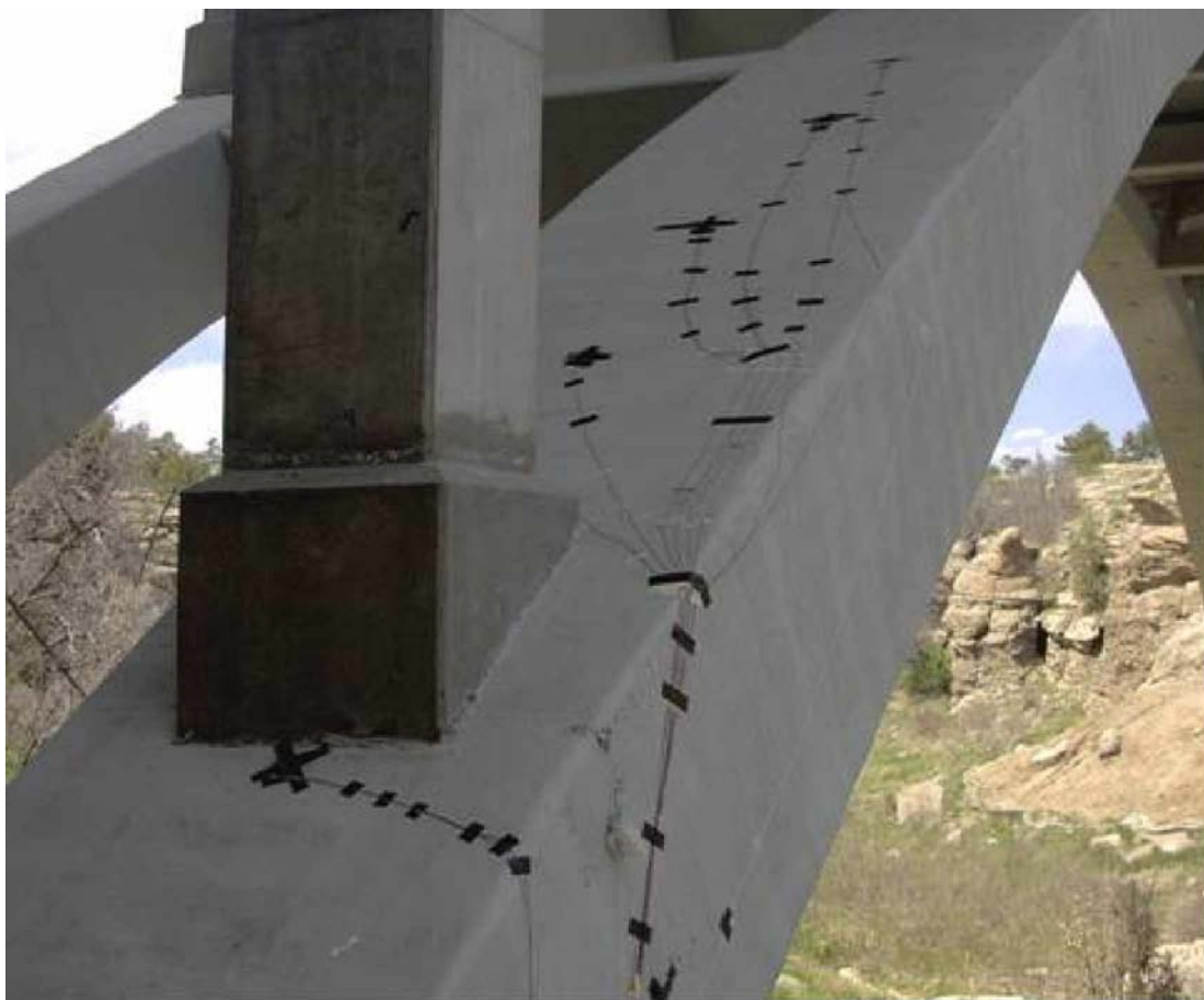
Figure 3-7 Wiring of strain gages - Extrados (Back)
