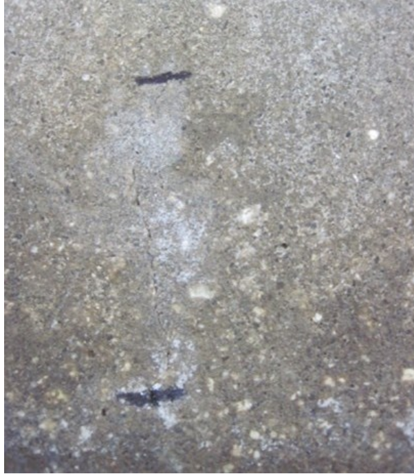
Figure 8-11. Crack observed on the front side of sample STD3-MMFX-B before termination.
