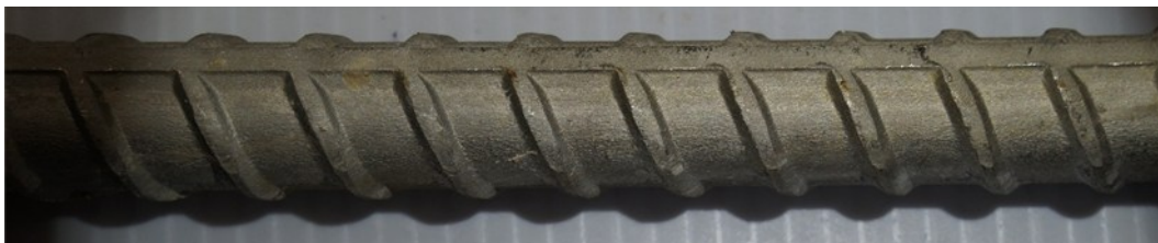
Figure 7-21. Closeups of pitting corrosion on 316SS rebar.
