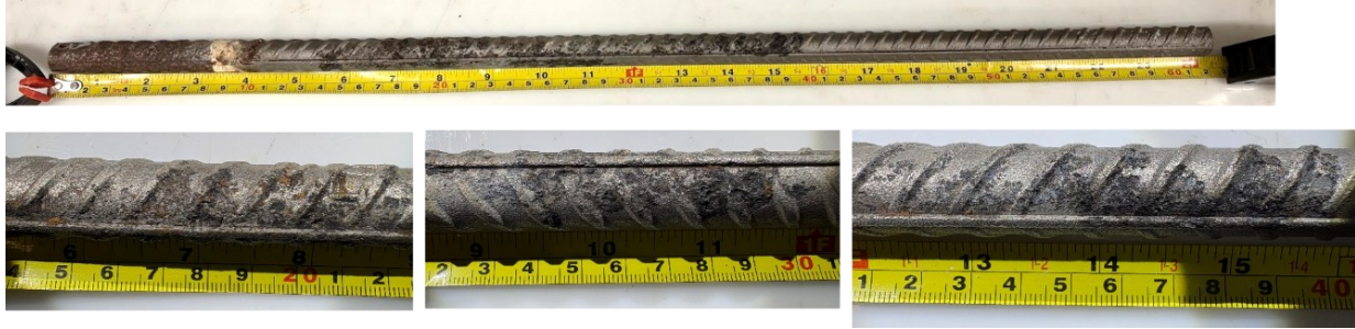
Figure 8-49. STD3-3CR12-E - full length of rebar 3 and notable areas of corrosion damage.
