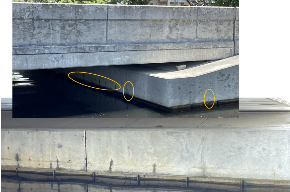
Figure 6-5. South side of the bridge under the deck, showing several cracks (moisture allows observation).
