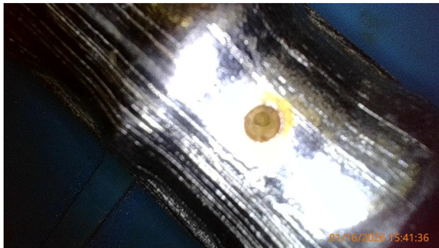
Figure 7-62. Hole 1 on bottom side of rebar A of sample CSDB-CT2-1.
