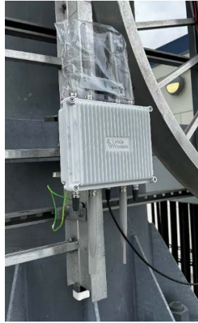
Figure 4-14: RSU mounted on the side of the gantry structure.
