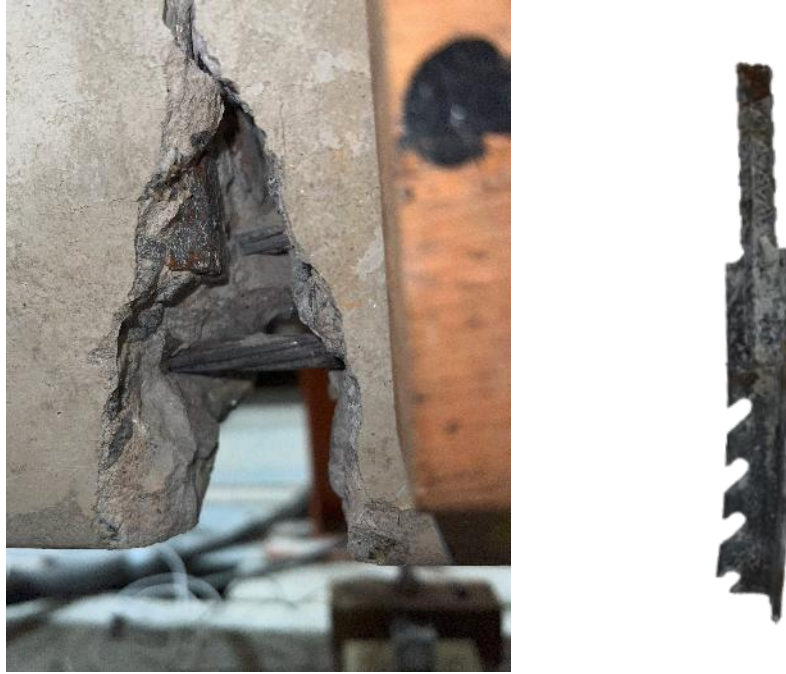
Figure 8.9 Hold-down device and ruptured strands (left) and hold-down device (right).
