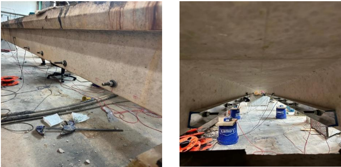
Figure 4.4 Aluminum channels through-bolted with steel threaded rods.
