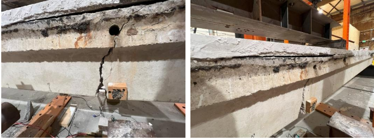
Figure 8.8 Flexural cracking and LMC delamination after 619,028 cycles.
