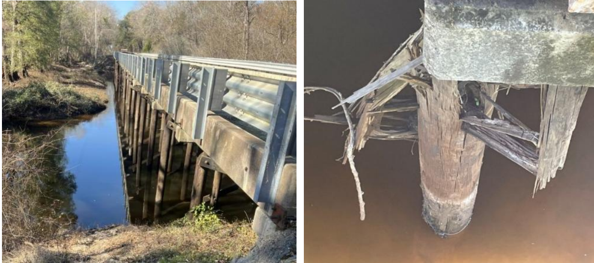
Figure 9.5 Four-hole swamp bridge (left) and pile failure (right).
