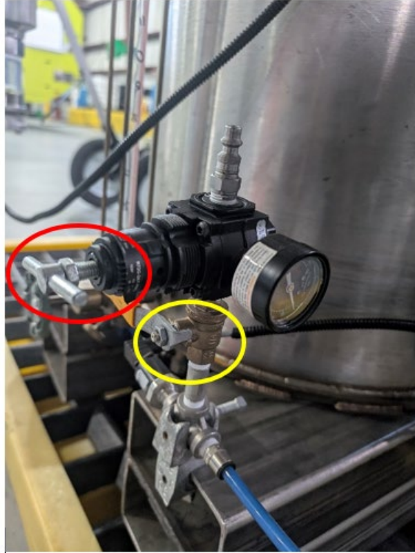
Figure 18. Compressed Air Valve (circled in yellow) and Compressed Air Regulator (adjustment circled in red)
