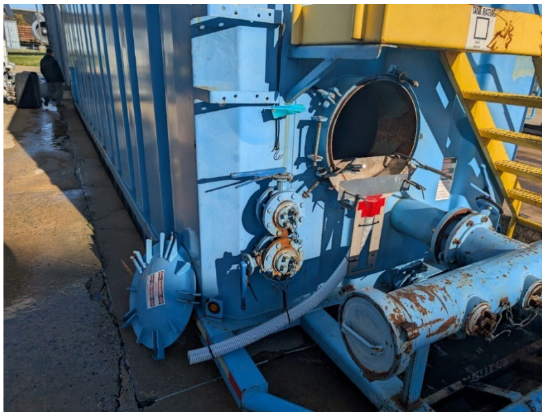
Figure 8. Sample Collection Board and Tubing Affixed to the Wall Tank Manway
