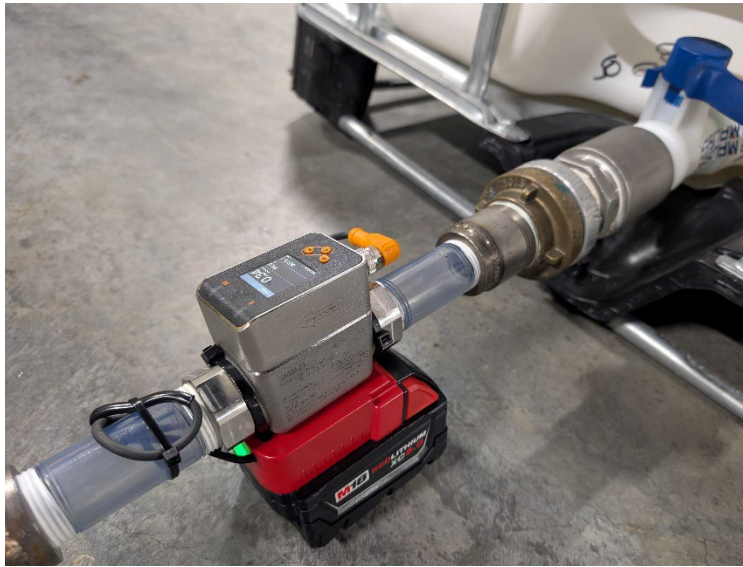
Figure 11. IFM Efector, Inc. SM8621 Flow Meter Affixed to IBC
