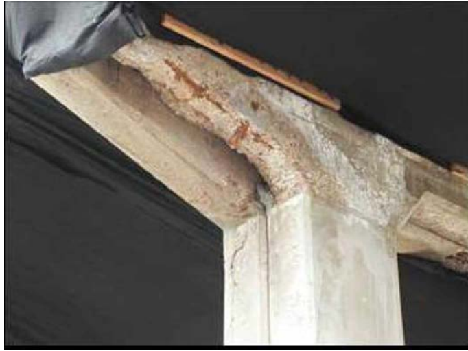
Figure 2-2 The corrosion-induced spalling in the spandrel column
