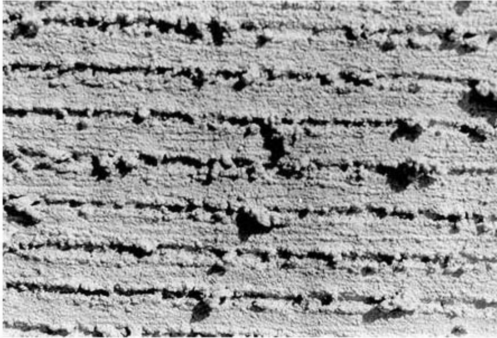
Photo 4: Popcorn-like mortar balls (longitudinal tining)
