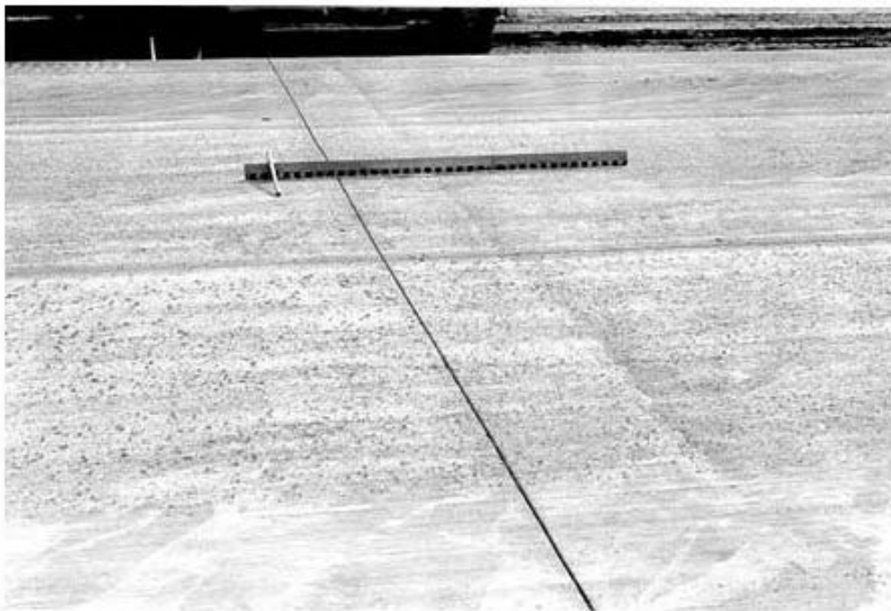
Photo 5: Transverse indentation of plastic concrete
