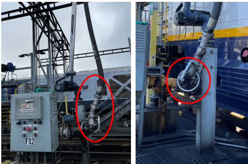
Figure 5. Example refueling receptacle diesel locomotives
