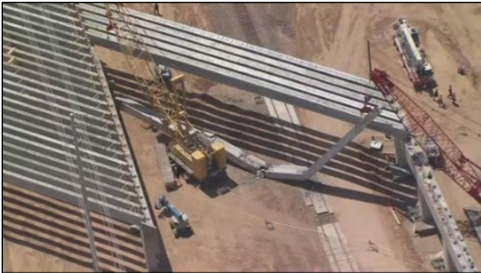
Figure 2.15. Lifting failure, VDOT (2022)
