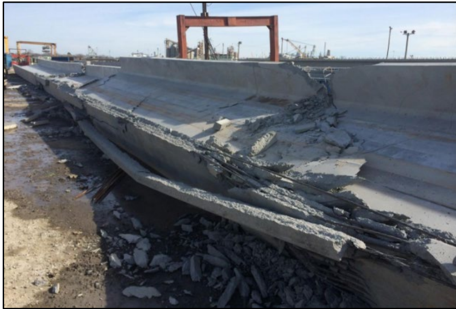
Figure 2.13. Failure during fabrication, VDOT (2022)
