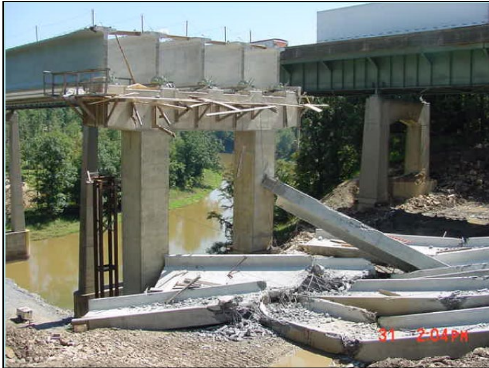
Figure 2.16. Failure of erected girders, courtesy of TxDOT
