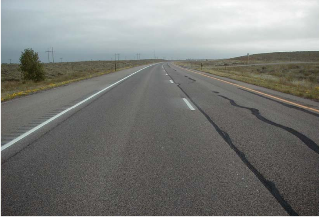
Figure 11. Typical WB Condition (9/24/05)
