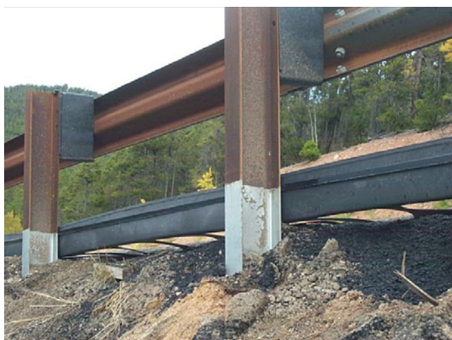
Figure 24. Inadequate base for the DFC.
