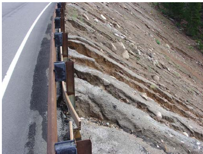
Figure 5. Severe erosion can occur very rapidly.
