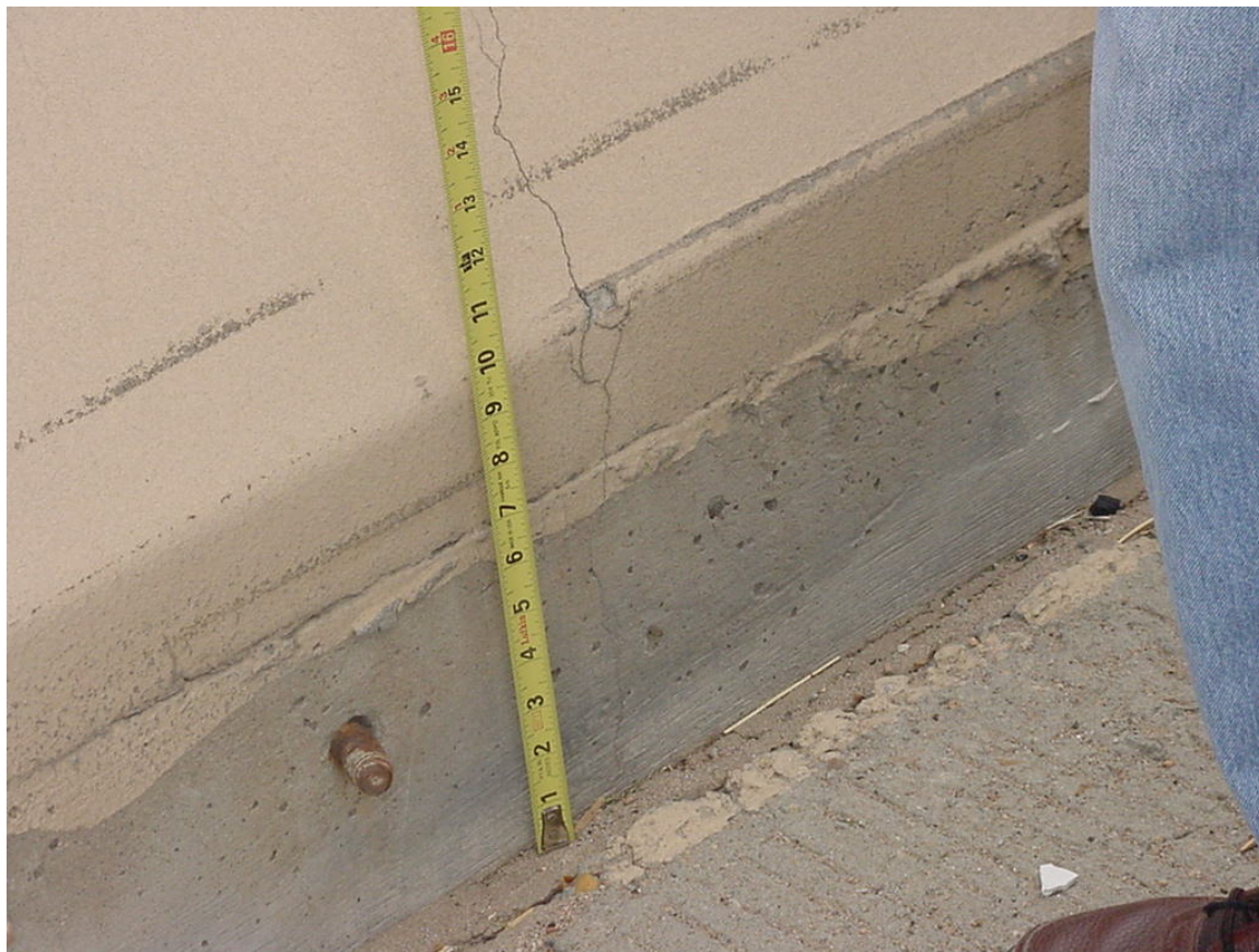
Figure C.5. A Settlement of 6" Between the Roadway and the Bridge Concrete Rail: North-East Side of Structure E-17-SW in Region 6.
