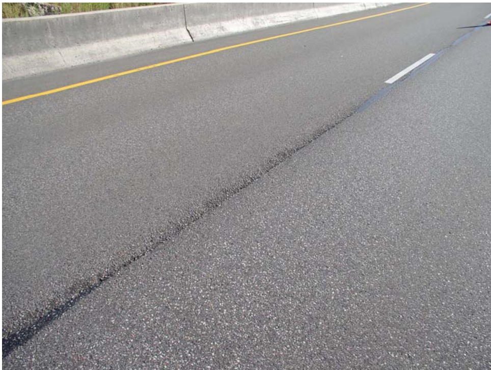
Figure 13. Raveling at Longitudinal Joint
