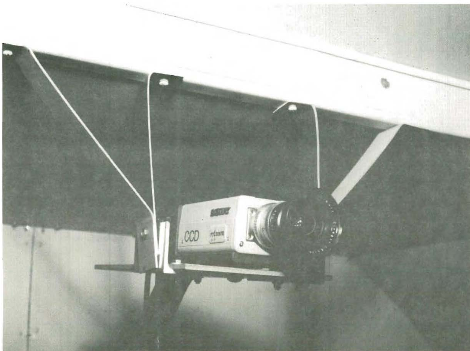
FIGURE 2.3.1-2 AFT VIDEO CAMERA
