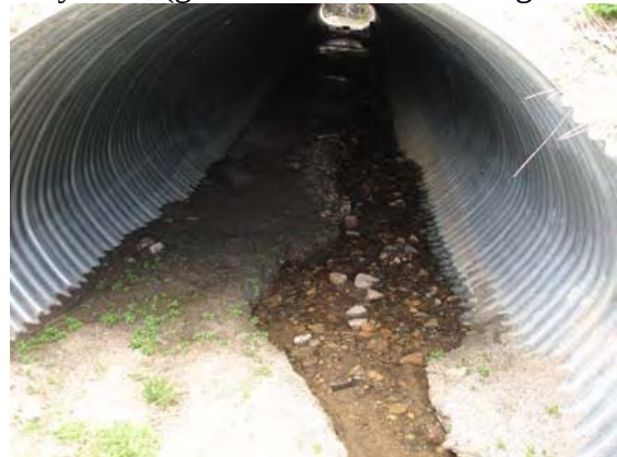
May 2006 (ground water flow through tunnel)
