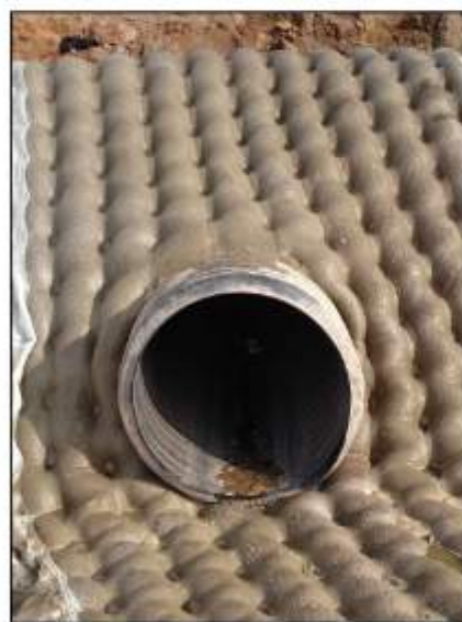
FILTER POINT CULVERT CUTOUT PICTURE JUST FOR REFERENCE
