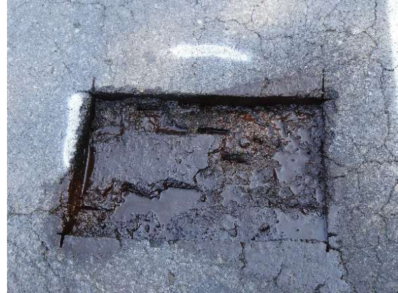
(b) Tack Coat Applied on a Rectangular Pothole Surface
