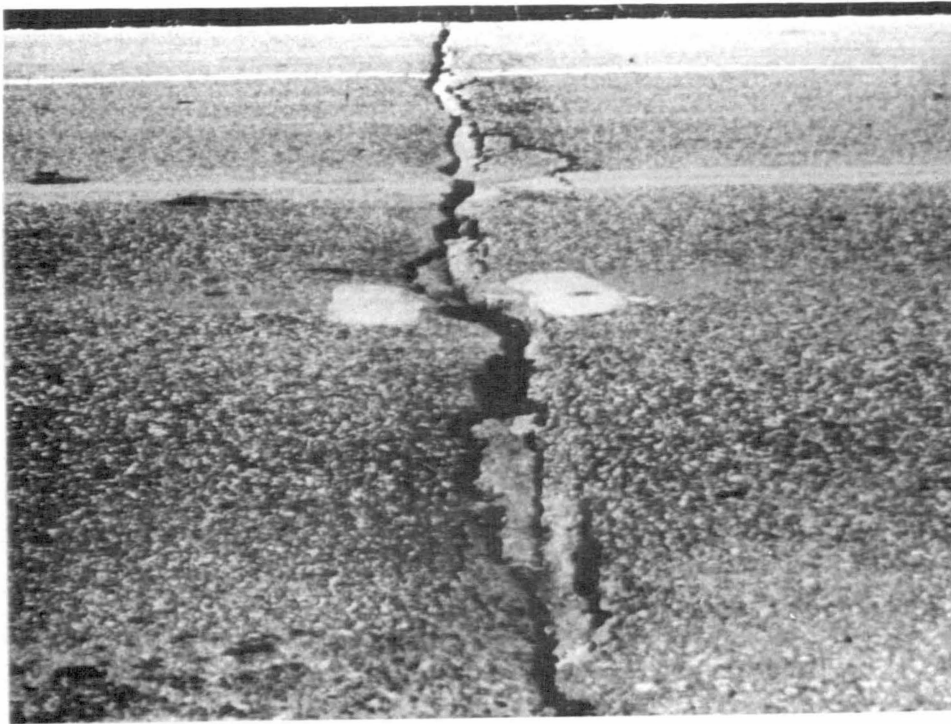
(Figure 1) Badly deteriorated transverse crack.
