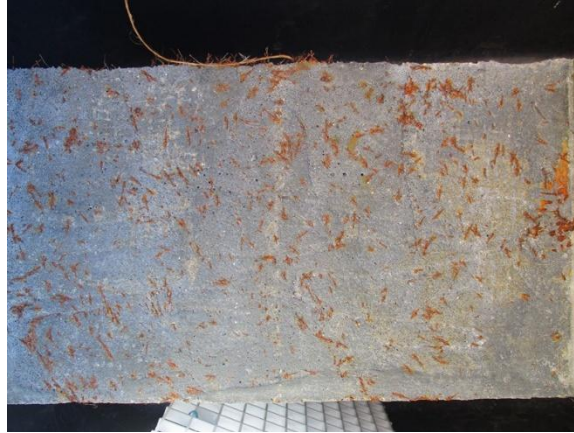
Photo 7.6. Exposed fiber corrosion.
