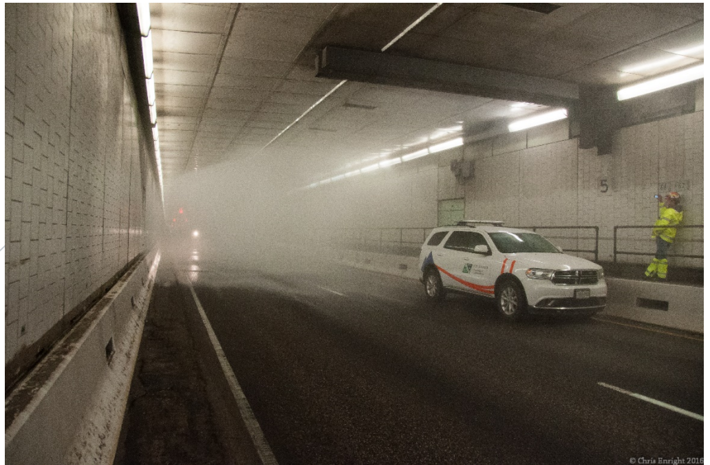
SPRINKLER OPERATION IN EISENHOWER TUNNEL
