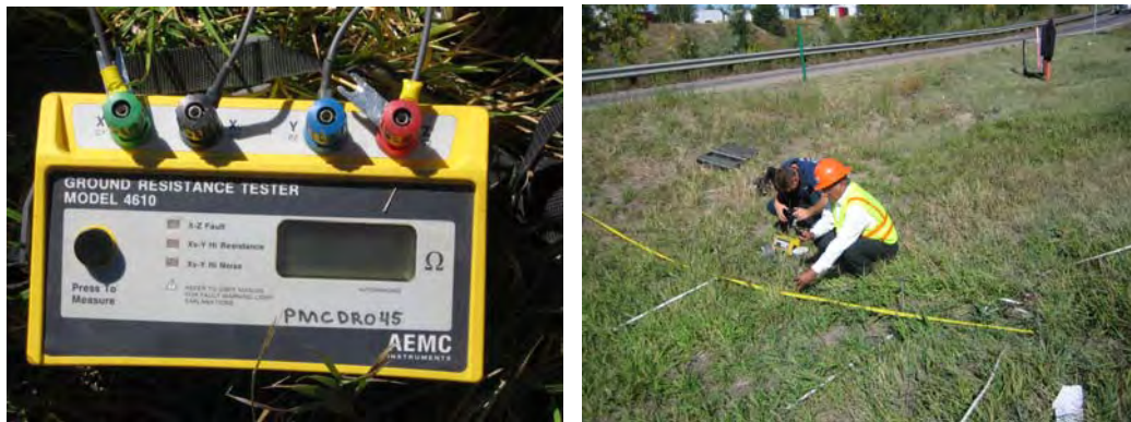
Figure 1. Soil resistivity testing by ASTM G57-95a
