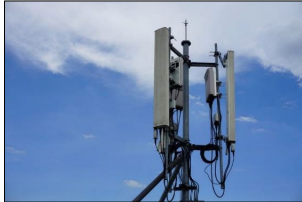
Figure 48. Example of a typical three-sectored cellular tower with panel antennas
