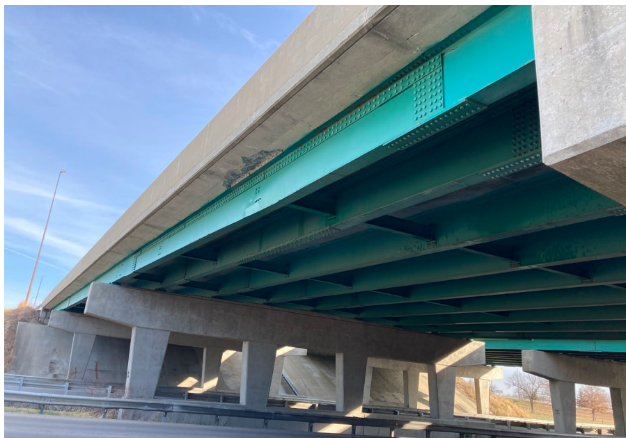
Figure 61. Photo. Overall view of damage to IDOT Bridge SN 084-0014. Girder 18, the front fascia girder, was damaged in the strike (the impact occurred from left to right).
