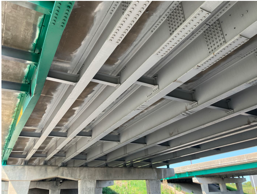
Figure 65. Photo. Overall bottom view of damage to IDOT Bridge SN 084-0077; Girder 19 is the left fascia girder (the impact occurred from left to right).
