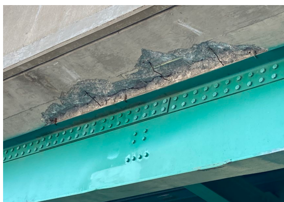
Figure 62. Photo. Close-up view of damage to the concrete deck above the impact point on the fascia girder of IDOT Bridge SN 084-0014 Girder 18.
