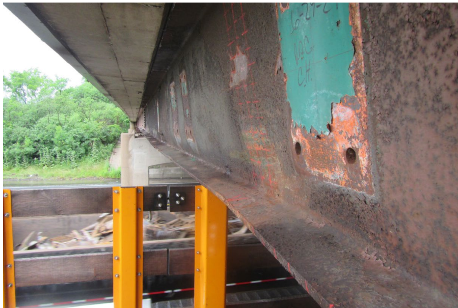
Figure 69. Photo. Damage to IDOT Bridge SN 016-0918 Girder 1, looking toward the center of the span. Red marks drawn on the web indicate the longitudinal location of impact, while bolt holes and green paint indicate directional sign attachment points.
