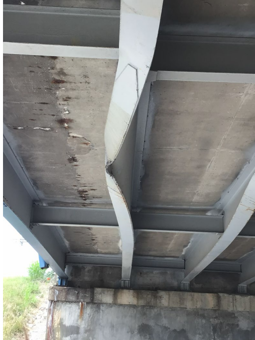
Figure 73. Photo. Bottom view of damage to IDOT Bridge SN 041-0067 Girder 6, showing excessive displacement.
