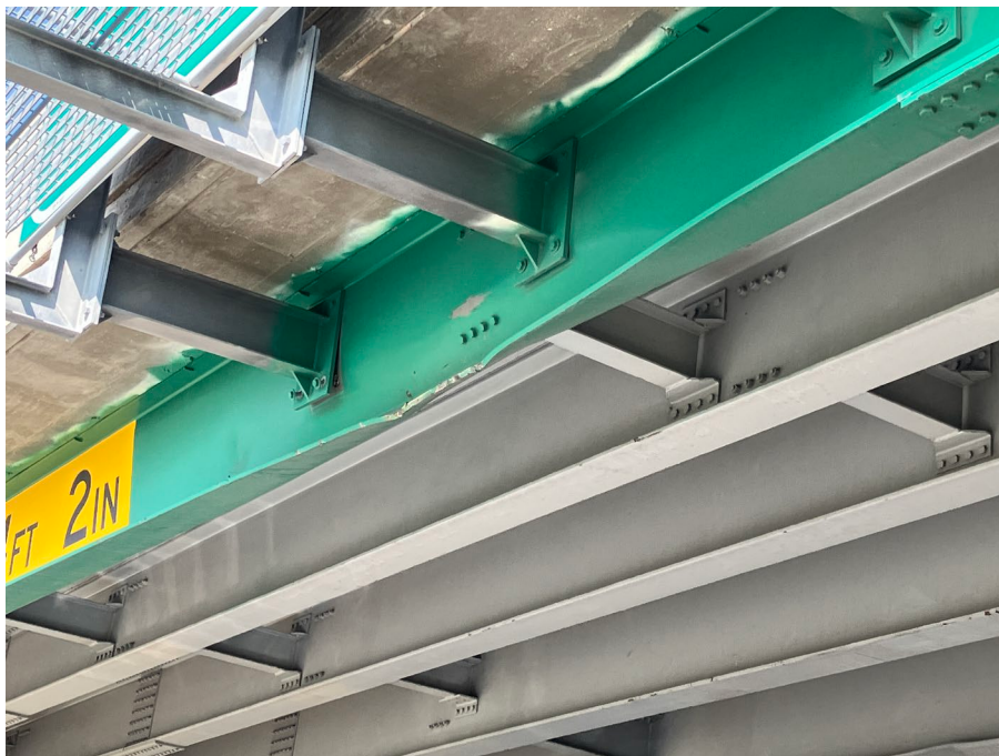
Figure 66. Photo. Front view of damage to IDOT Bridge SN 084-0077 Girder 19.
