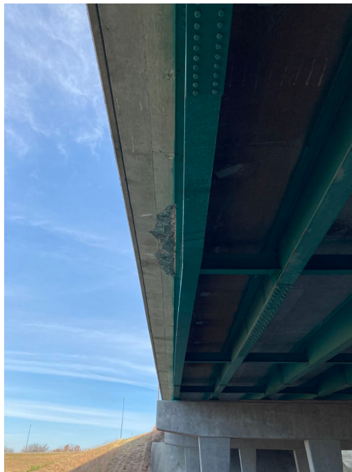
Figure 64. Photo. Bottom view of damage to IDOT Bridge SN 084-0014 Girder 18, looking toward the center pier. The girder is displaced toward the right.
