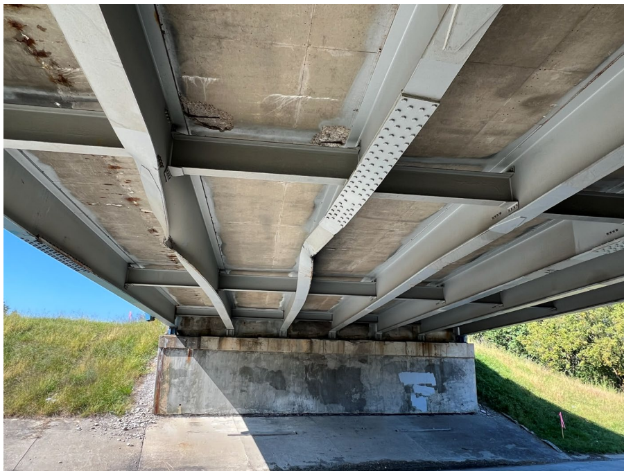
Figure 72. Photo. Overall bottom view of damage to IDOT Bridge SN 041-0067. Girder 6 is the first interior girder from left and was damaged most severely.
