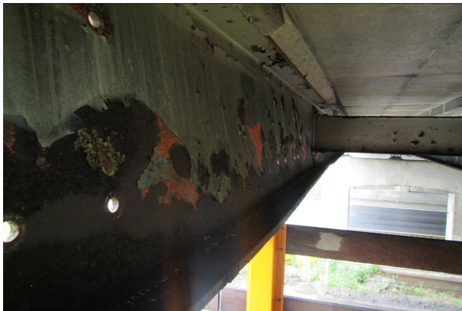
Figure 70. Photo. Back view of damage to IDOT Bridge SN 016-0918 Girder 1, looking toward the center of the span. Paint on the back of the girder is peeling.
