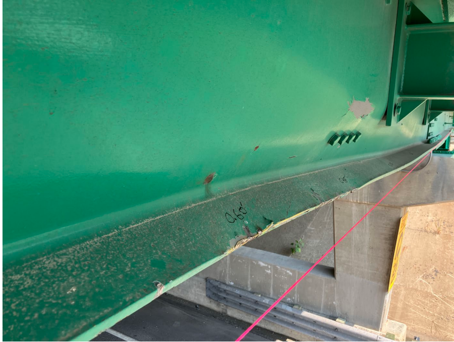
Figure 67. Photo. Close-up view near the impact point on IDOT Bridge SN 084-0077 Girder 19. Small nicks and scratches are visible. (The stringline reference is pink.)
