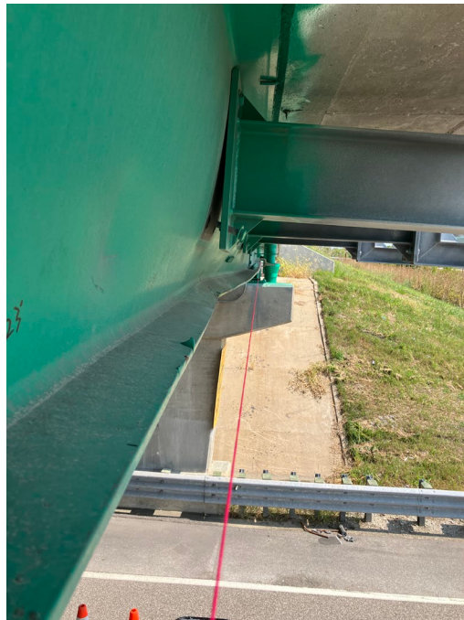
Figure 68. Photo. Longitudinal view of damage to IDOT Bridge SN 084-0077, looking away from the center pier. (The stringline reference is pink.)
