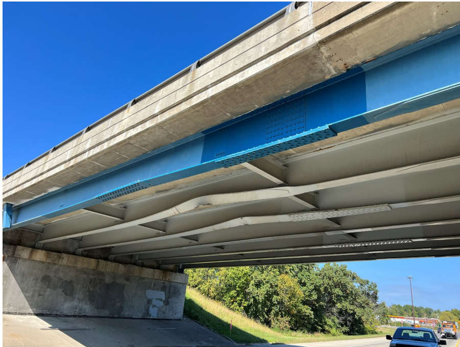
Figure 71. Photo. Overall view of damage to IDOT Bridge SN 041-0067. Girder 6 is the first interior girder from front. (Several girders were damaged by the oversized load shown in Figure 1.)
