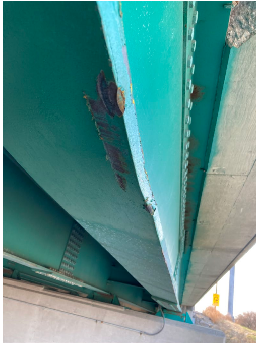
Figure 63. Photo. Close-up view of the impact point on IDOT Bridge SN 084-0014 Girder 18. Small nicks and scratches are visible.
