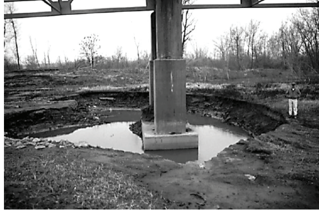
Figure 1 Local scouring a bridge pier after flow event.
