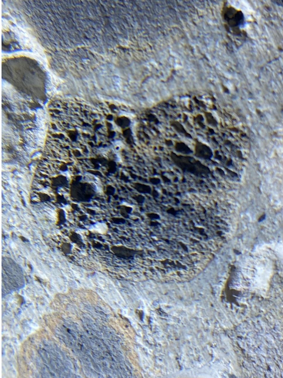
Figure E.25 Aggregate in core 5 of lightweight concrete deck at bridge F-792 (2).
