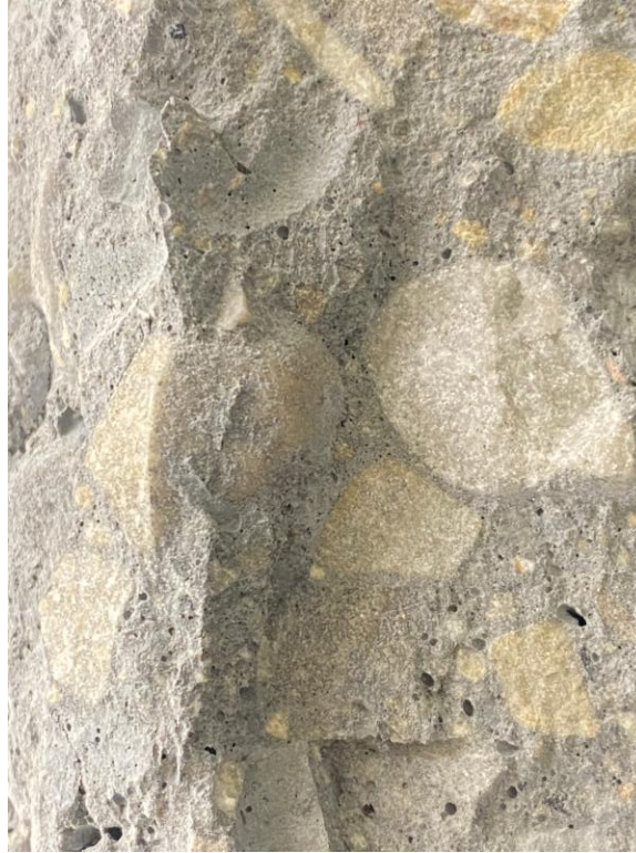
Figure 4.12 Normal-weight concrete fracture face.
