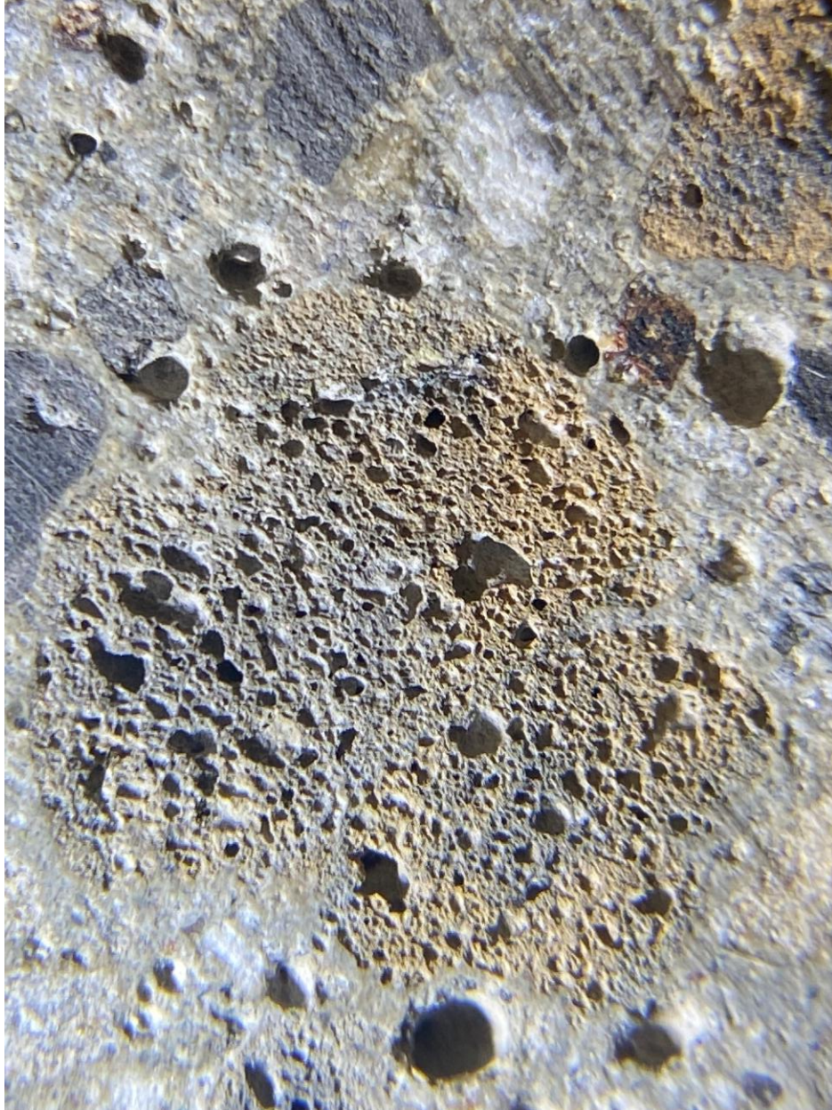
Figure E.16 Aggregate in core 1 of lightweight concrete deck at bridge F-792 (1).
