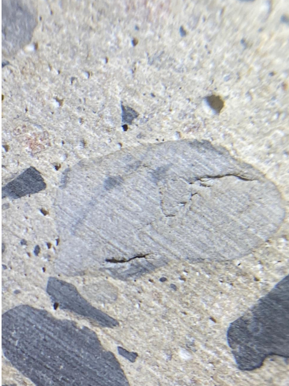
Figure E.15 Aggregate in core 5 of lightweight concrete deck at bridge C-1011.
