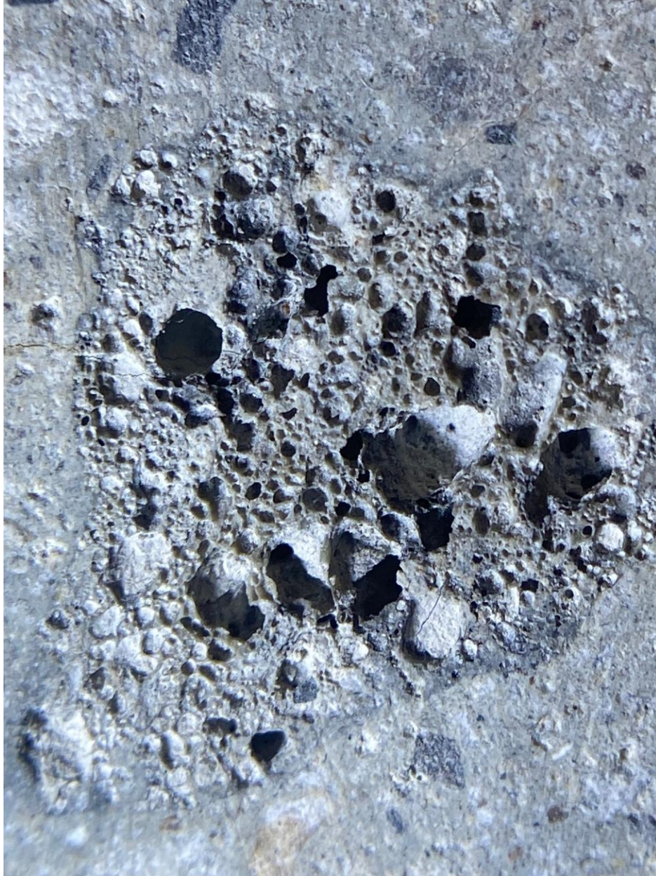
Figure E.21 Aggregate in core 4 of lightweight concrete deck at bridge F-792 (1).
