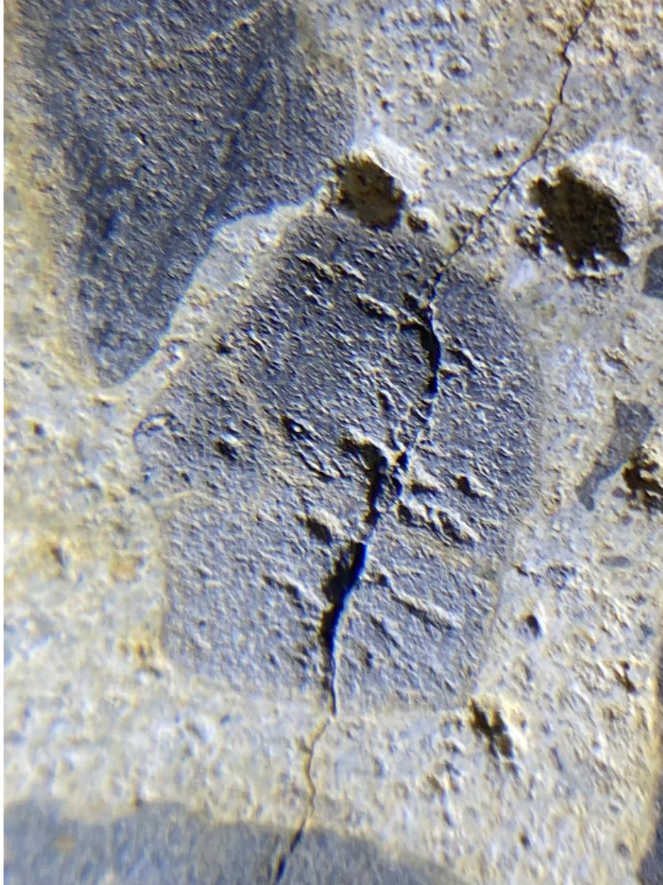
Figure E.23 Aggregate in core 4 of lightweight concrete deck at bridge F-792 (3).
